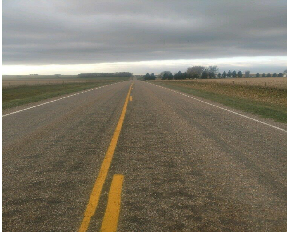
Figure 142. Appearance of Otta seal surface two months post construction – long view with pavement markings
