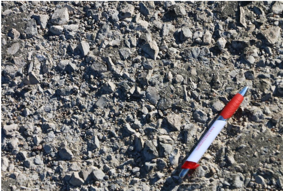
Figure 139. Appearance of Otta seal surface two weeks post construction of test section using limestone
