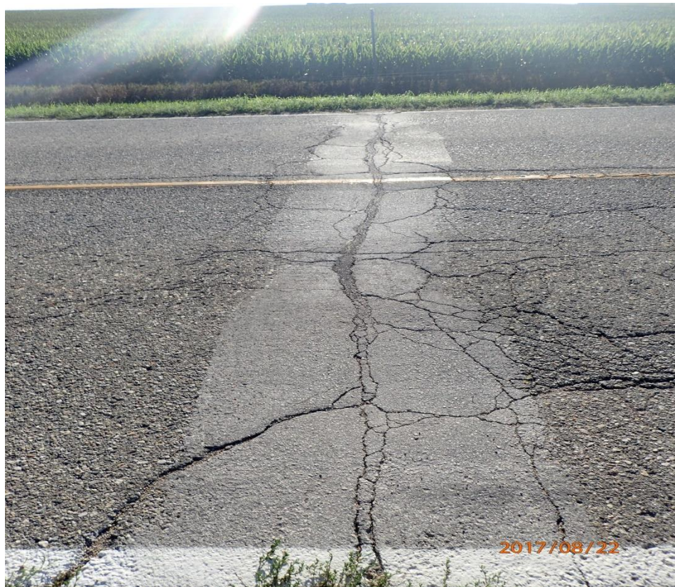
Figure 91. Existing transverse cracking
