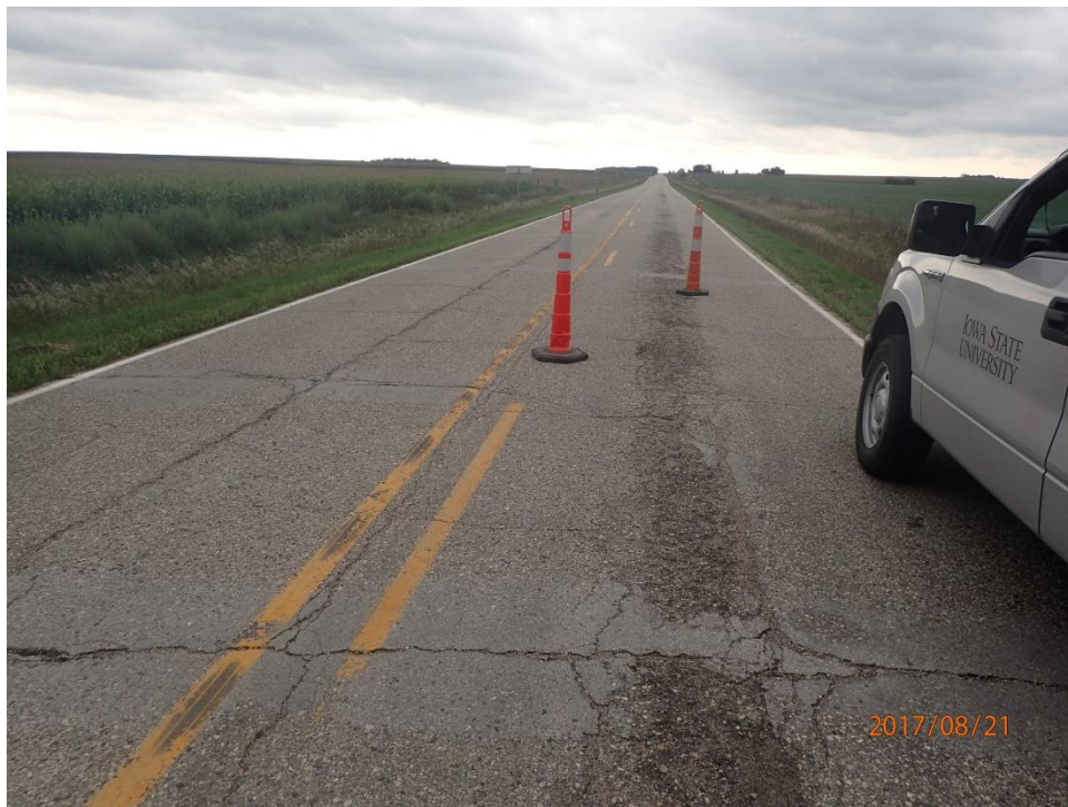
Figure 89. Longitudinal and transverse cracking present before implementing Otta seal in Cherokee, Iowa
