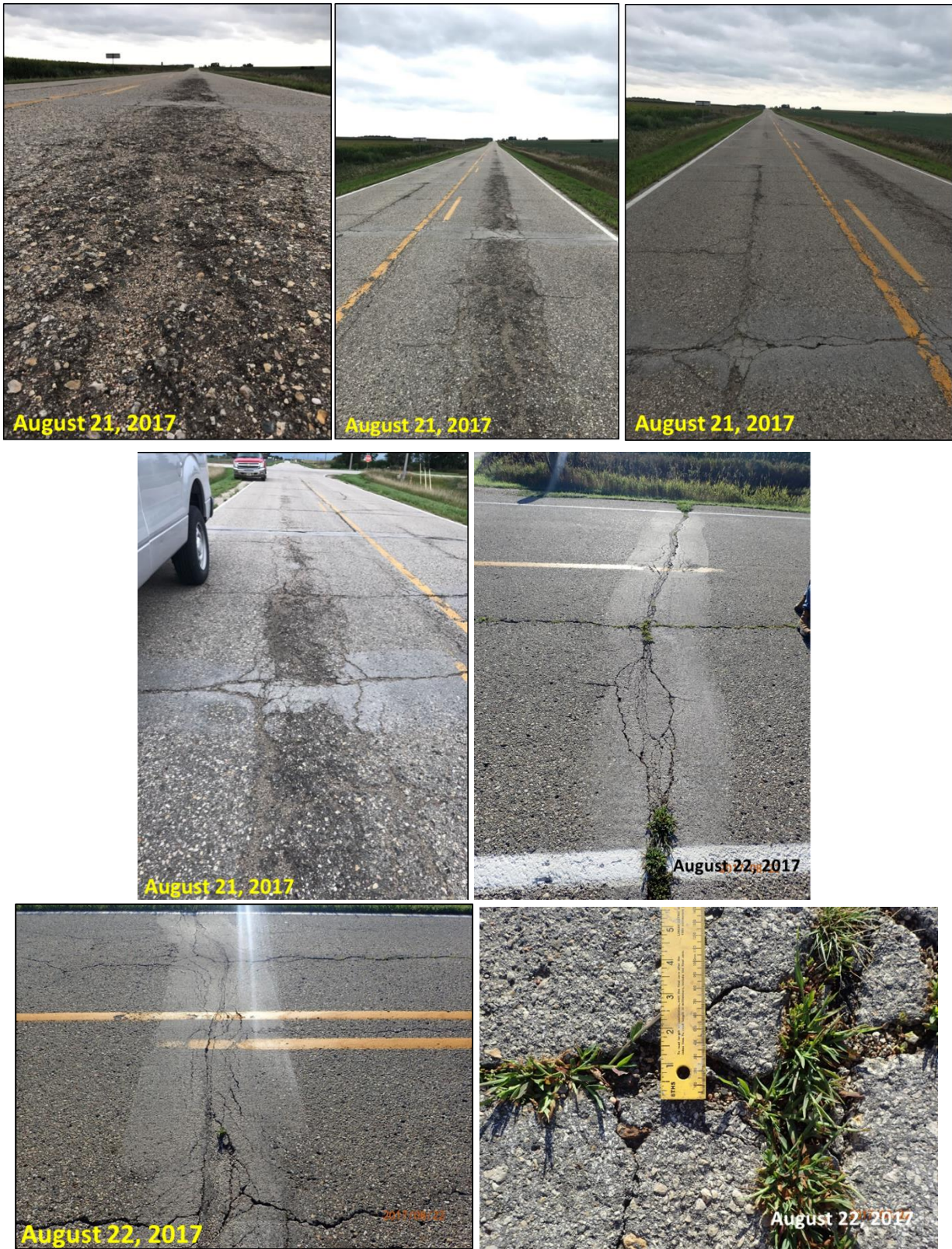
Figure 36. Various types of distresses observed on CR L-40 Otta seal project site prior to any surface treatment, August 21–22, 2017
