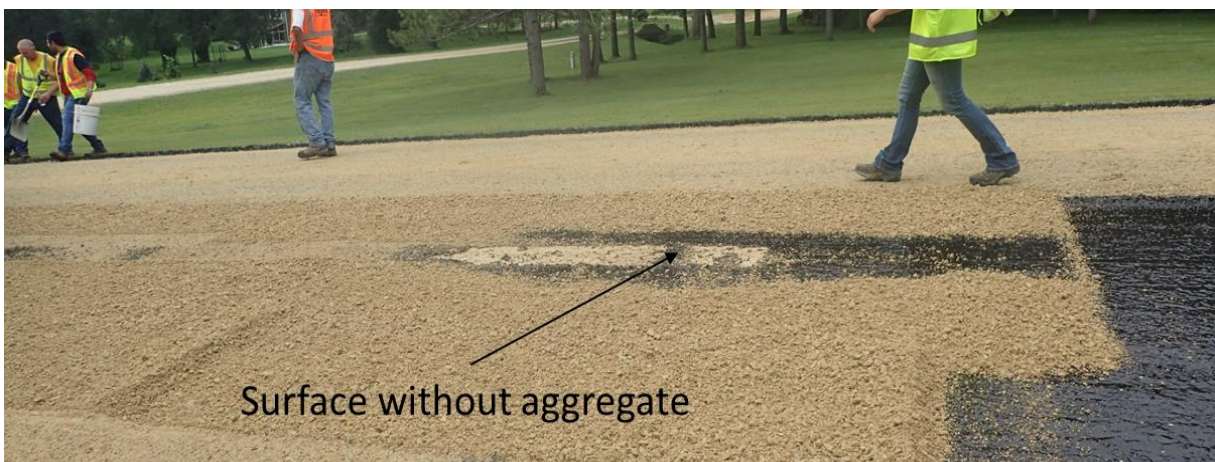
Figure 27. Aggregate not well distributed on some spots of the surface
