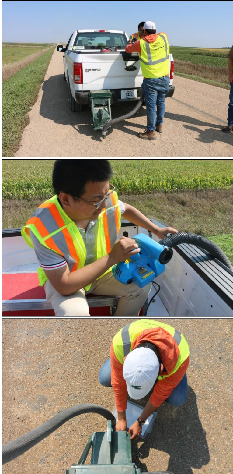
Figure 60. Three steps of installing the dustometer tester: installing the dustometer on a truck, preparing the vacuum, and placing filter paper in the tester
