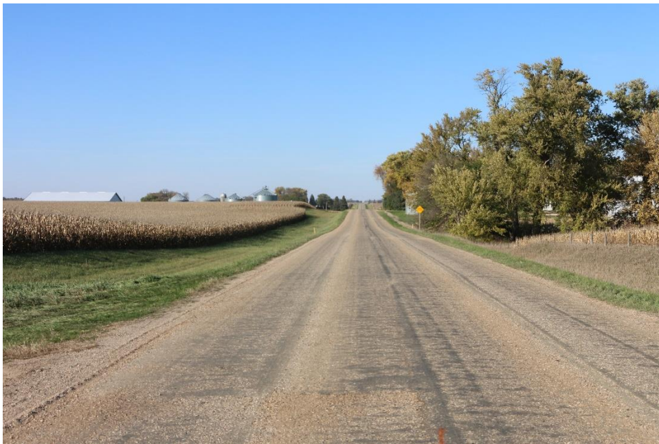
Figure 137. Appearance of Otta seal two weeks post construction, showing surface changed to darker color
