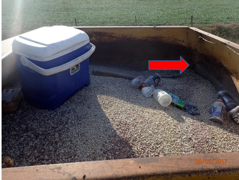
Figure 54. Roller was not filled to the required weight for first layer construction
