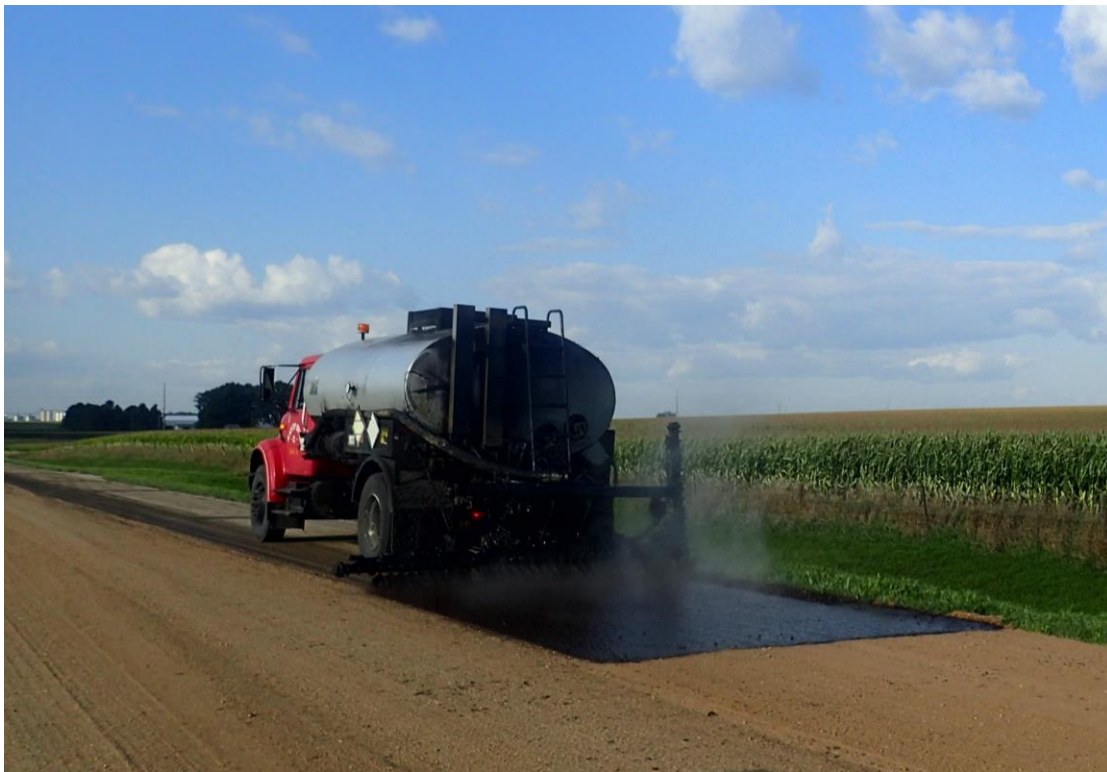
Figure 44. The emulsion asphalt binder HFMS-2s applied for Otta seal construction on CR L-40, Cherokee County, Iowa
