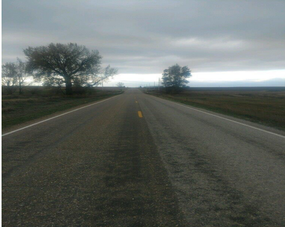
Figure 144. Appearance of Otta seal surface two months post construction, showing dark surface
