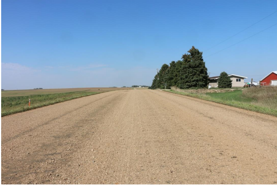
Figure 130. Appearance of Otta seal two days post construction showing dark areas near lane center
