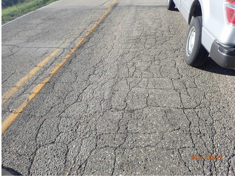
Figure 90. Severe alligator cracking on the HMA surface
