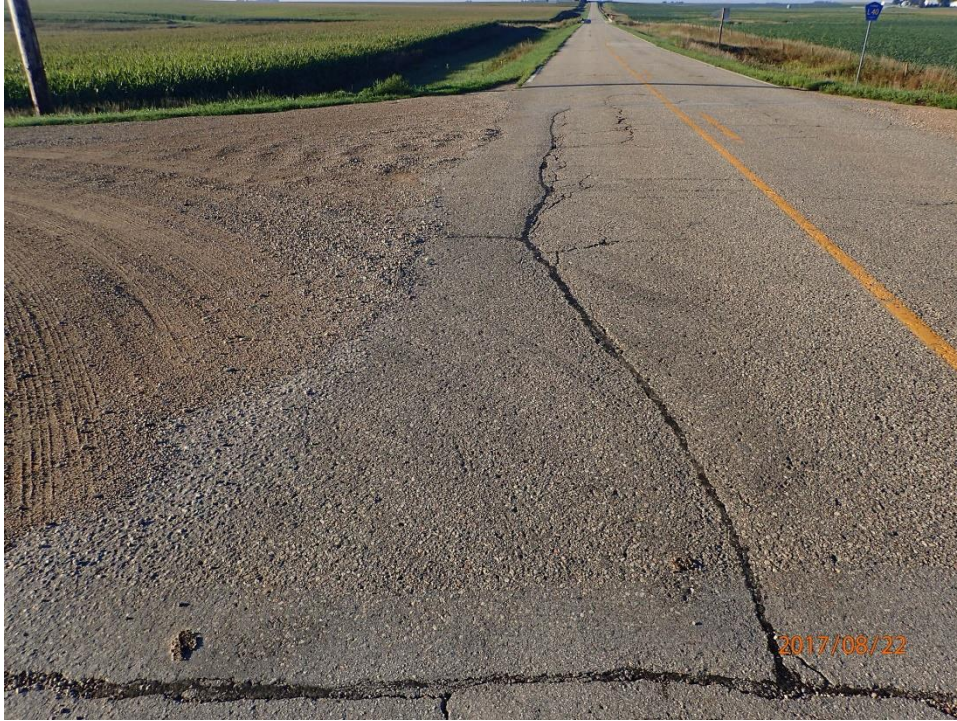
Figure 94. Existing cracking at intersection area
