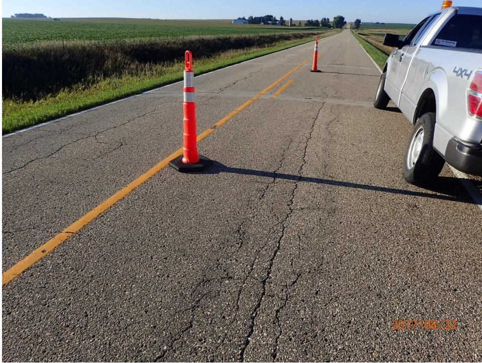
Figure 92. Existing longitudinal cracking
