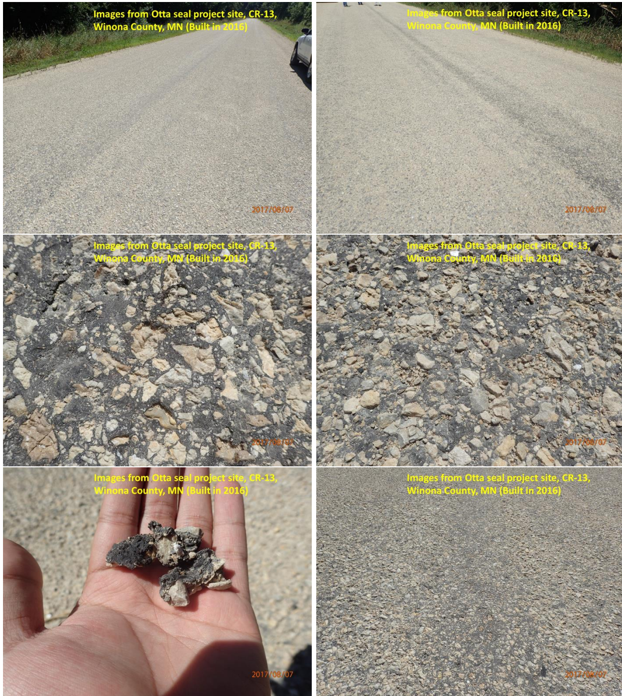
Figure 34. Performance of Otta seal on CSAH 13 Winona County, Minnesota
