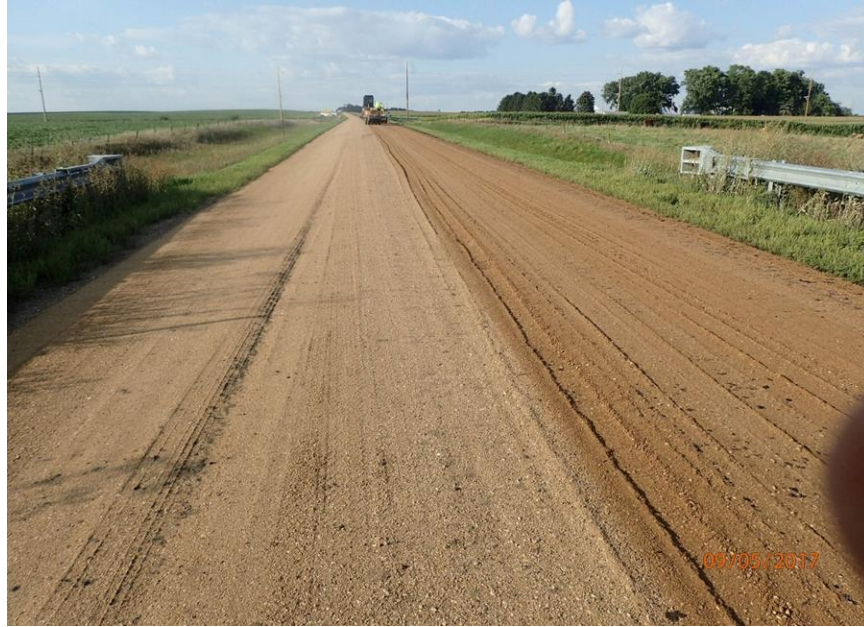
Figure 53. Partially compacted (left) versus uncompact (right) lanes
