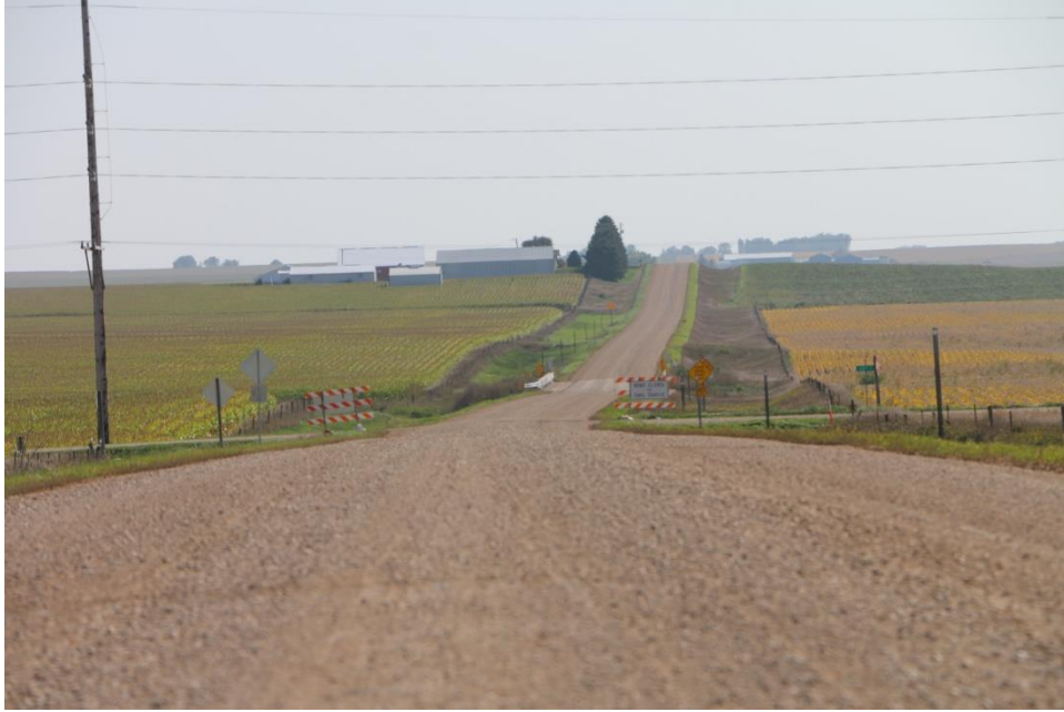
Figure 126. Long view of the second layer Otta seal two days post construction
