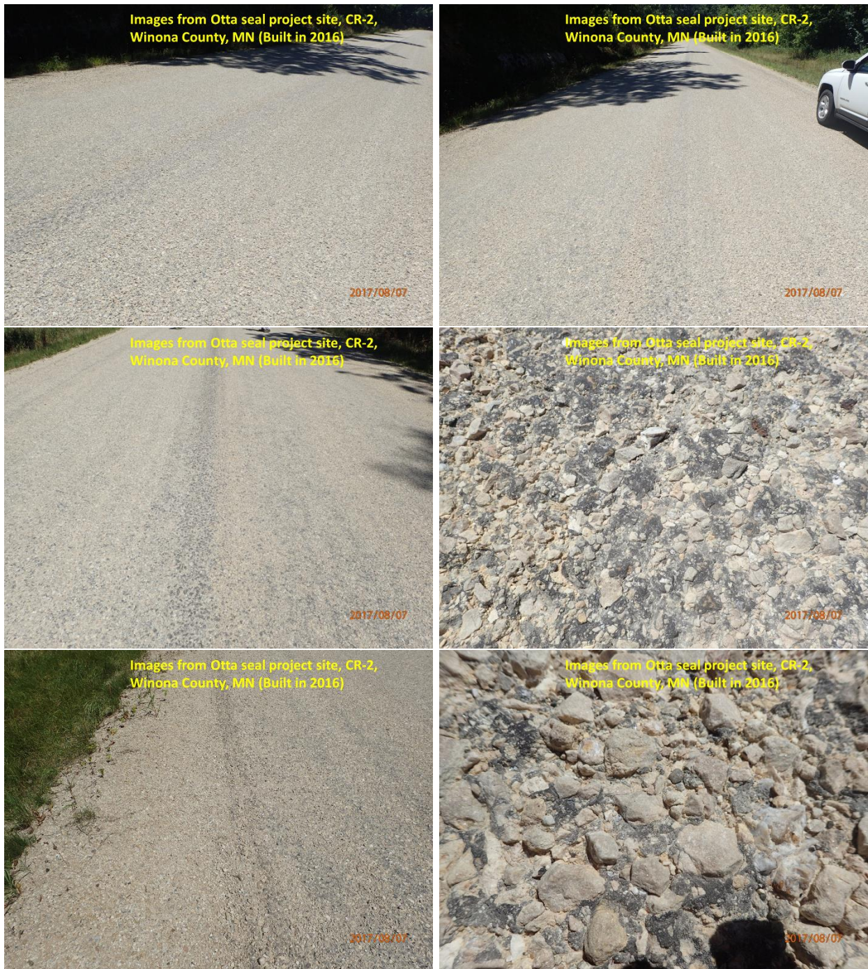
Figure 33. Performance of Otta seal on CSAH 2 Winona County, Minnesota
