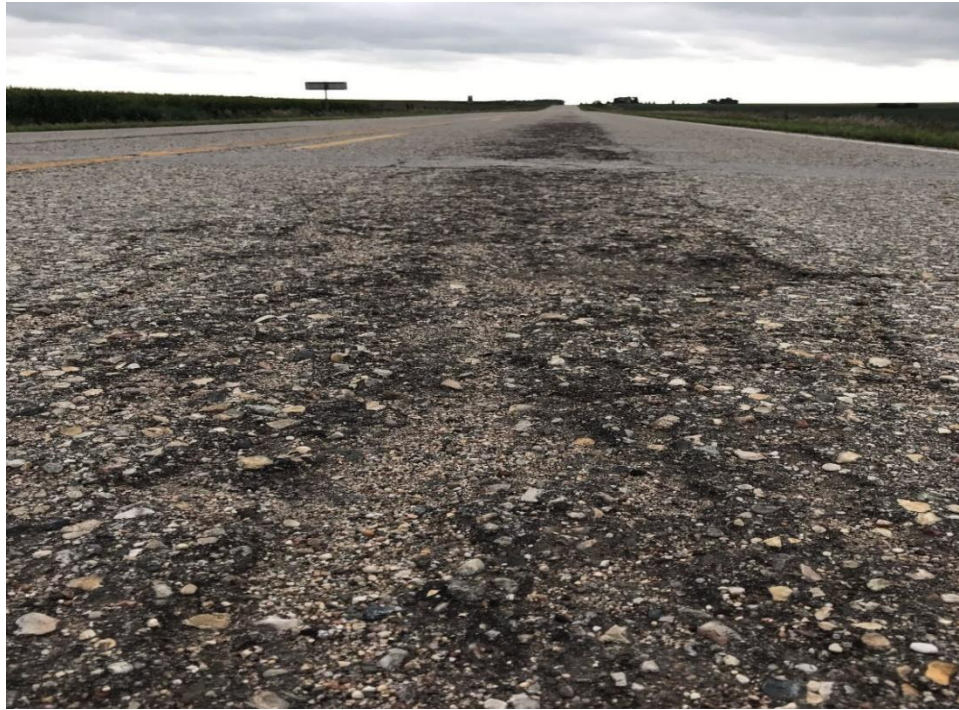
Figure 88. Condition of the road surface before implementing Otta seal in Cherokee, Iowa
