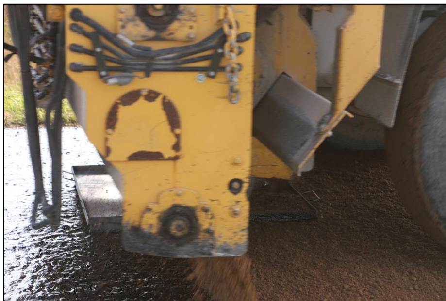
Figure 57. Aggregate spreader passing over the pan, with aggregates falling on the pan
