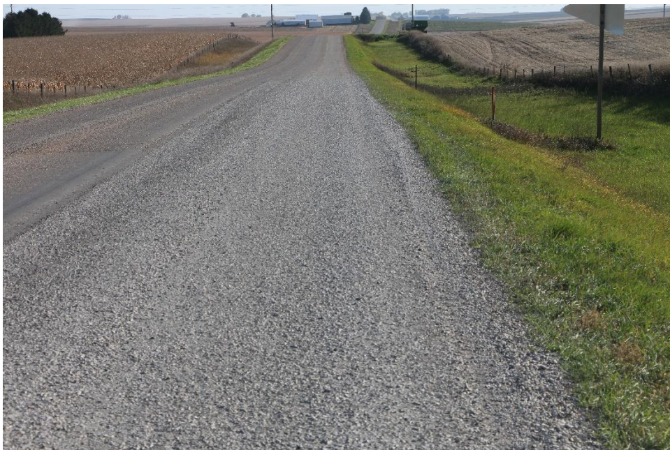
Figure 135. Appearance of Otta seal two weeks post construction showing one test section
