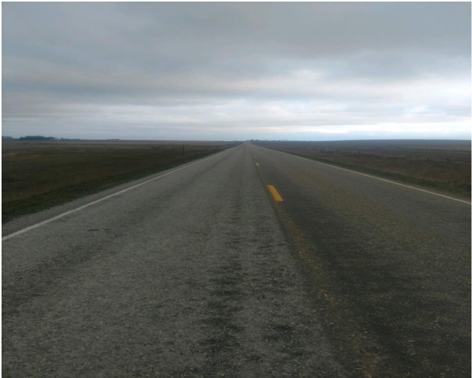
Figure 141. Appearance of Otta seal surface two months post construction
