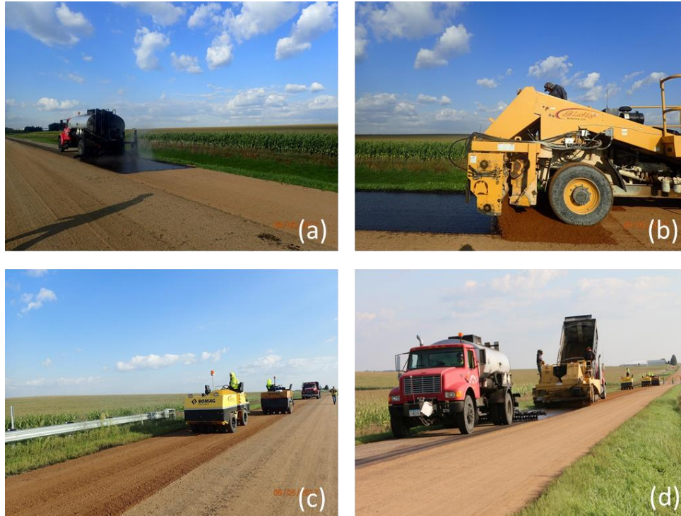
Figure 55. Construction of the second Otta seal layer: (a) binder spraying, (b) aggregate application, (c) rolling compaction, and (d) the complete process
