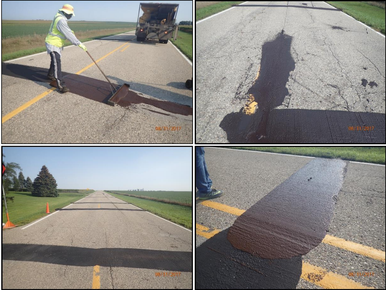
Figure 46. Slurry seal applied on the existing HMA pavement on CR L-40 before construction
