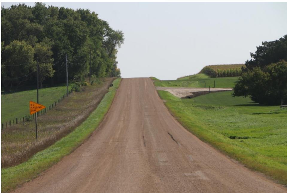
Figure 127. Appearance at a slope area of Otta seal two days post construction
