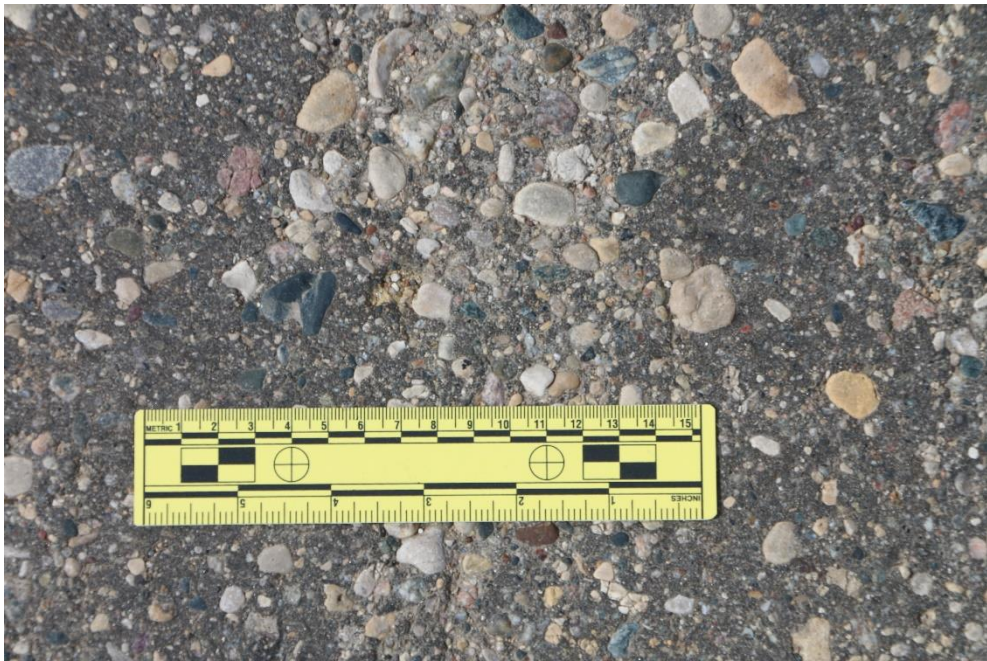
Figure 149. Appearance of Otta seal surface six months post construction, shown with scale
