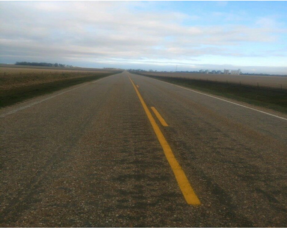
Figure 143. Appearance of Otta seal surface two months post construction, showing that surface continued to change to darker color
