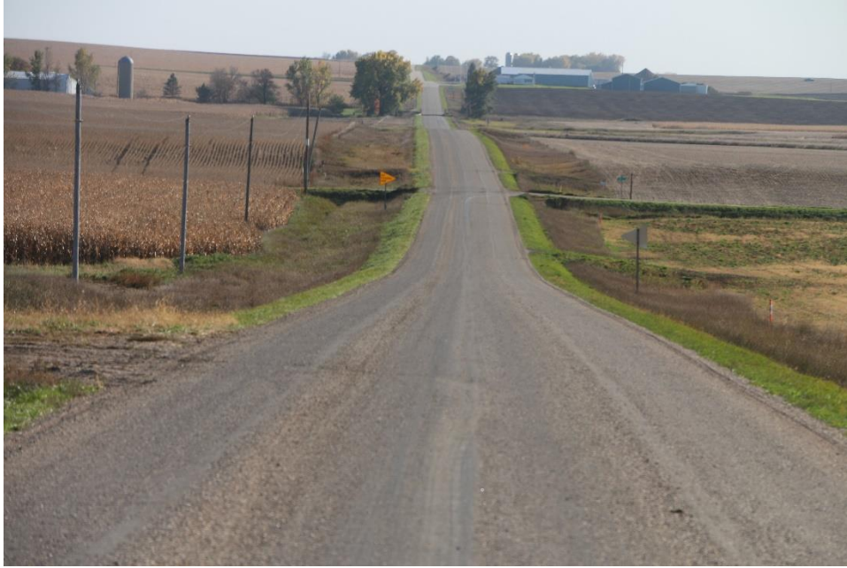
Figure 138. Appearance of Otta seal two weeks post construction, with lane center a lighter color than other areas
