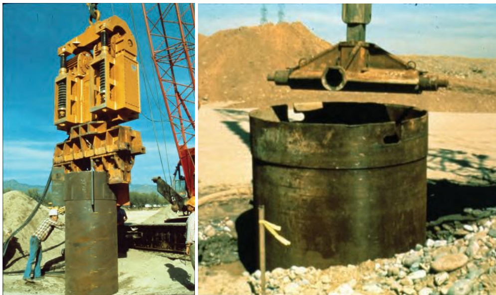
Figure 2.10 Use of a vibro-hammer (left) and twister bar (right) to advance casing (FHWA, 2010).
