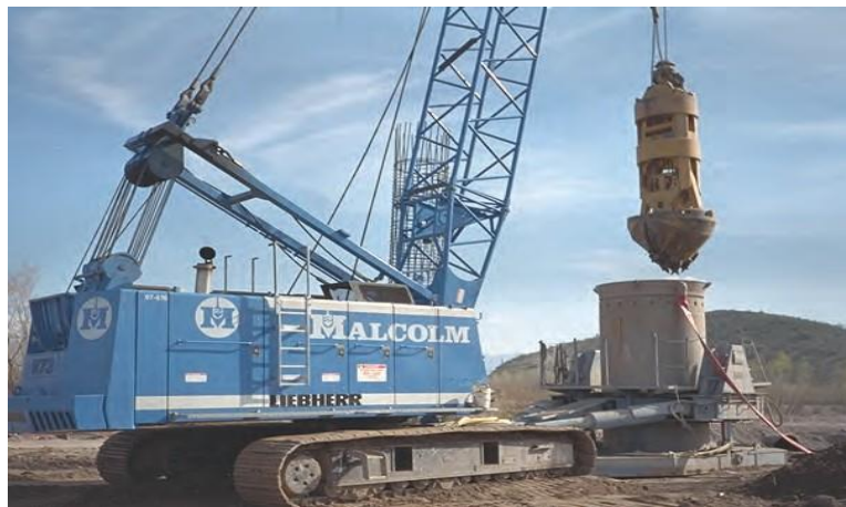
Figure 2.9 Oscillator rig used to advance segmental casing ahead of the excavation (FHWA, 2010).
