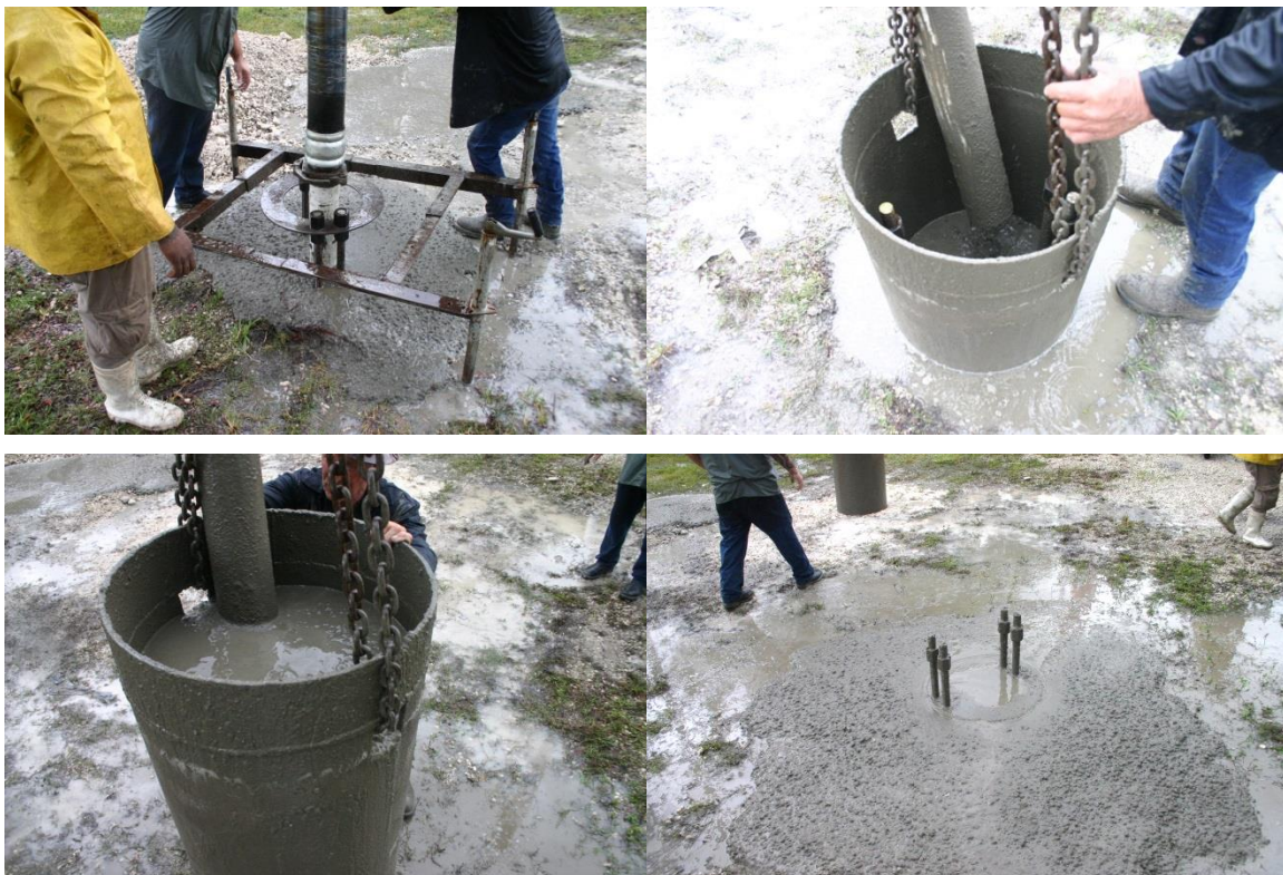
Figure 4.14 Concreting: over-pouring control shaft (top left); filling temporary casing with extra concrete (top right and bottom left) and after casing extraction (bottom right).
