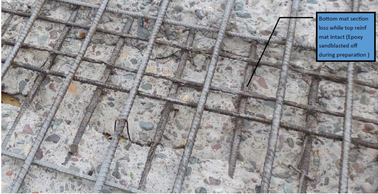
Figure D.1.26: Accelerated bottom mat (uncoated reinforcement) with localized corrosion in top mat (Epoxy-coated reinforcement).
