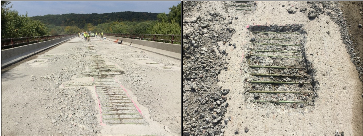
Figure D.1.23: In September 2017 the polymer overlay removed and patching was initiated. Photo on right shows epoxy-coated reinforcement corrosion at local defects that had spread. was Older epoxy coating processes were more susceptible to the coating debonding from the rebar.
