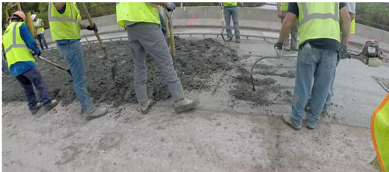
Figure D.1.25: A 2.5" thick low-slump concrete wearing course was placed to extend deck life until replacement. The center 12-foot wide pass consisted of a reinforced. The bridge was permanently load posted to reduce heavy truck loads.
