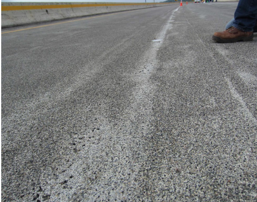
Figure 6.3 Br 09823 in Carlton County, MN, 2013 condition with some porosity due to unclean aggregate in 2009 TPO construction. Exhibiting a polished ridge along construction joint due to plows.
