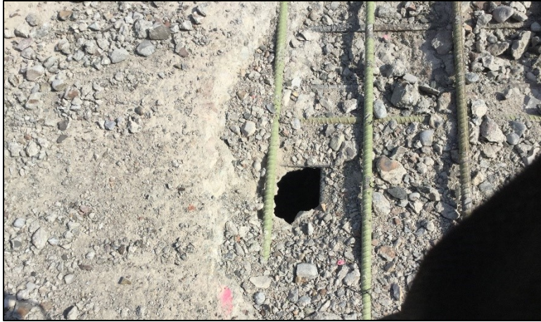
Figure D.1.24: Uncoated bottom reinforcement has corroded more rapidly and spalled off underside concrete cover, resulting in a slab that was prone to punch-through failure.
