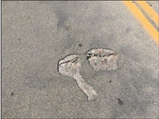
Figure D.1.22: Polymer overlay with debonding and concrete spalling progression.
