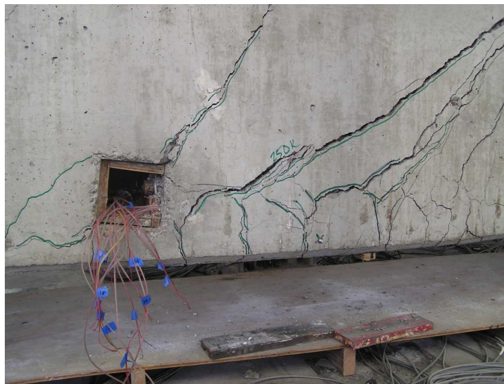
Fig. 4.10 – Typical anchorage cracking caused by slip of the cutoff bars
