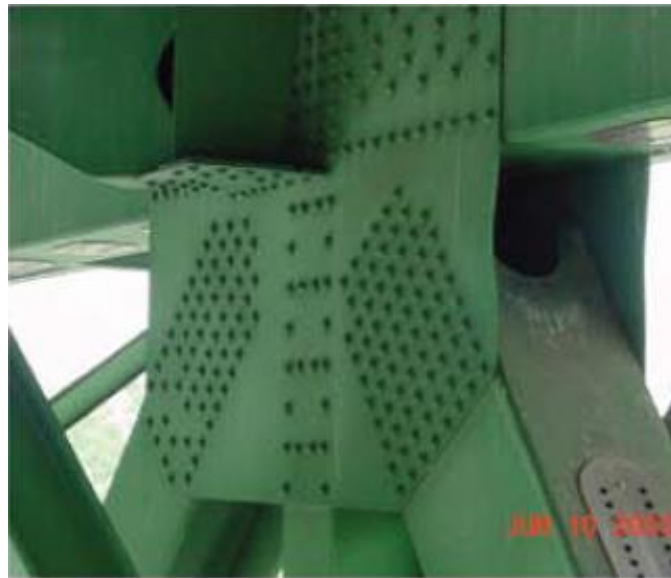
Figure 2.2 Photograph from 2003 of the failed gusset plate [1]
