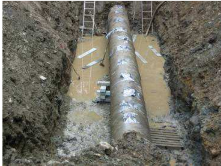
Figure 51. Water flooded the ditch, removing some of the dollies located at the 6 o'clock position.
