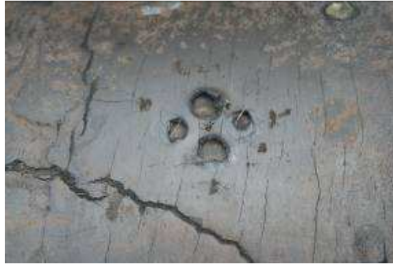
Figure 32. Pull-off adhesion measurements showing a failed spot near the defect.
