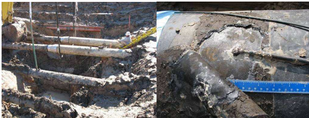
Figure 45. General and specific view of the excavation conducted by DNV COLUMBUS in Louisiana during January 2007
