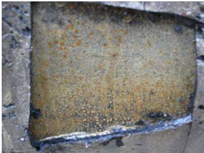
Figure 50. Removal of damaged coal tar coating prior to analysis on the areas adjacent to the defects.
