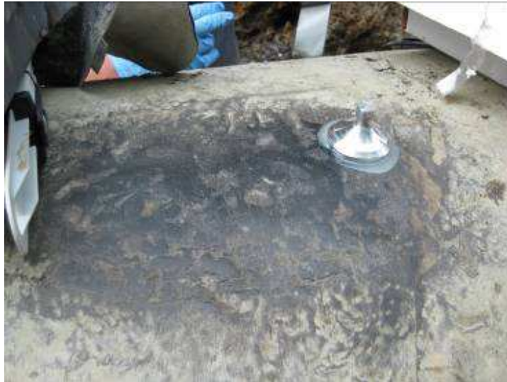
Figure 48. 50 mm dolly applied at the 12 o'clock position.
