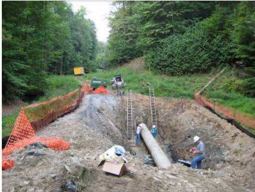
Figure 46. Pipe section before analysis.
