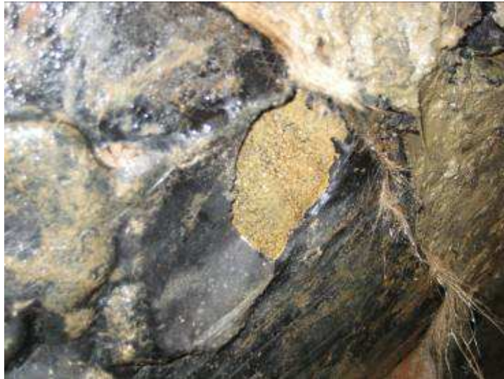
Figure 49. Signs of coating damaged were found at different locations.
