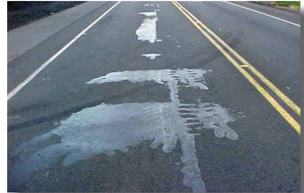
Figure 1 Pavement damage caused by infiltration of water
