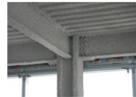
Sprayed Fire- Resistive Materials (SFRM)
