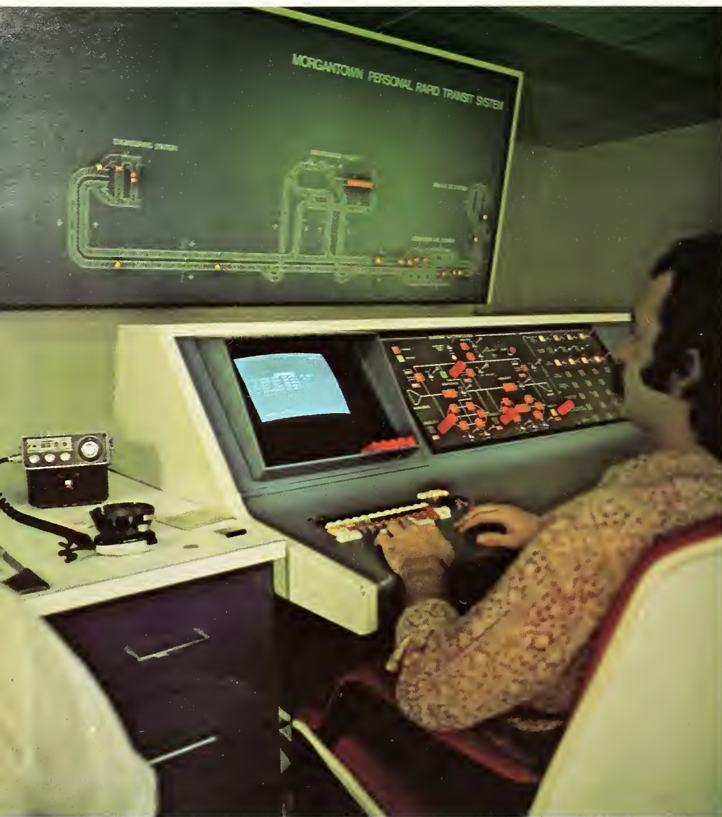
The electronic map and computer read-outs enable control room personnel to monitor the location and condition of every car.
