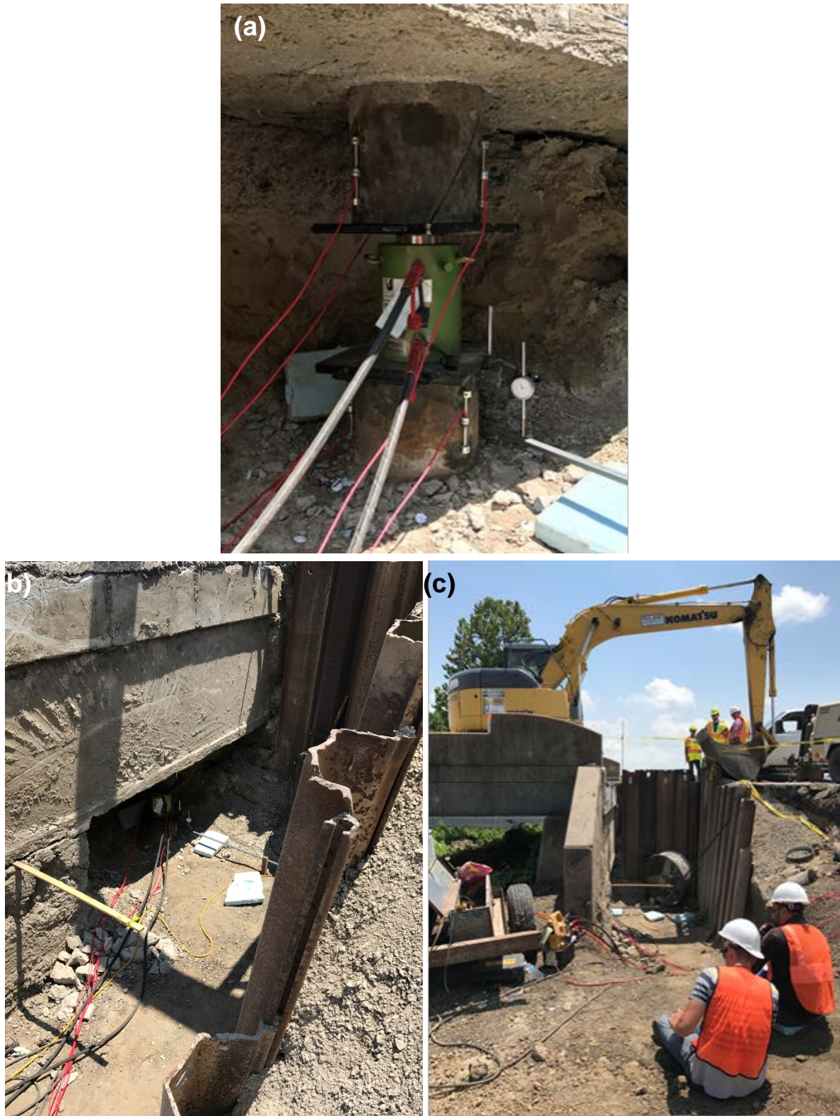
Figure 30: Photographs of CIP test pile load test: (a) hydraulic cylinder applies load while strain gages are used to measure load at the top of pile and dial gage measures displacement of the top of the pile; (b) view of test pile beneath existing bridge capping beam; and (c) backhoe is parked atop reaction beam to reduce loads in capping beam and reaction piles.
