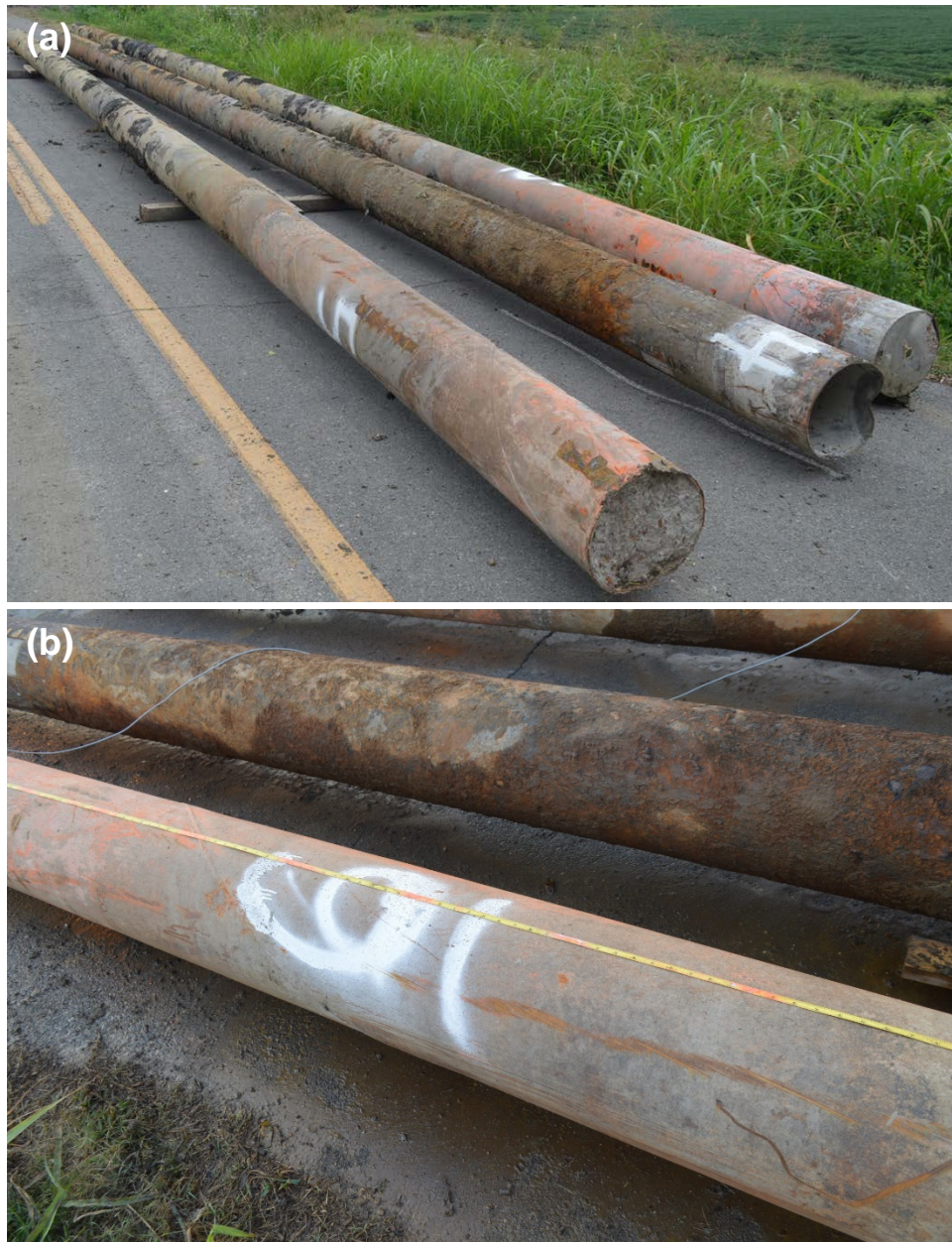
Figure 39: Photographs of exhumed CIP piles: (a) full length and (b) length of pile without surface corrosion in foreground and length of pile with surface corrosion in background. Note that although it is marked as Pile 6 this is Pile 8.
