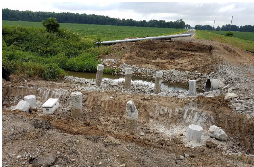
Figure 20: Overview photo of Route U site after bridge was removed and precast piles were cut.
