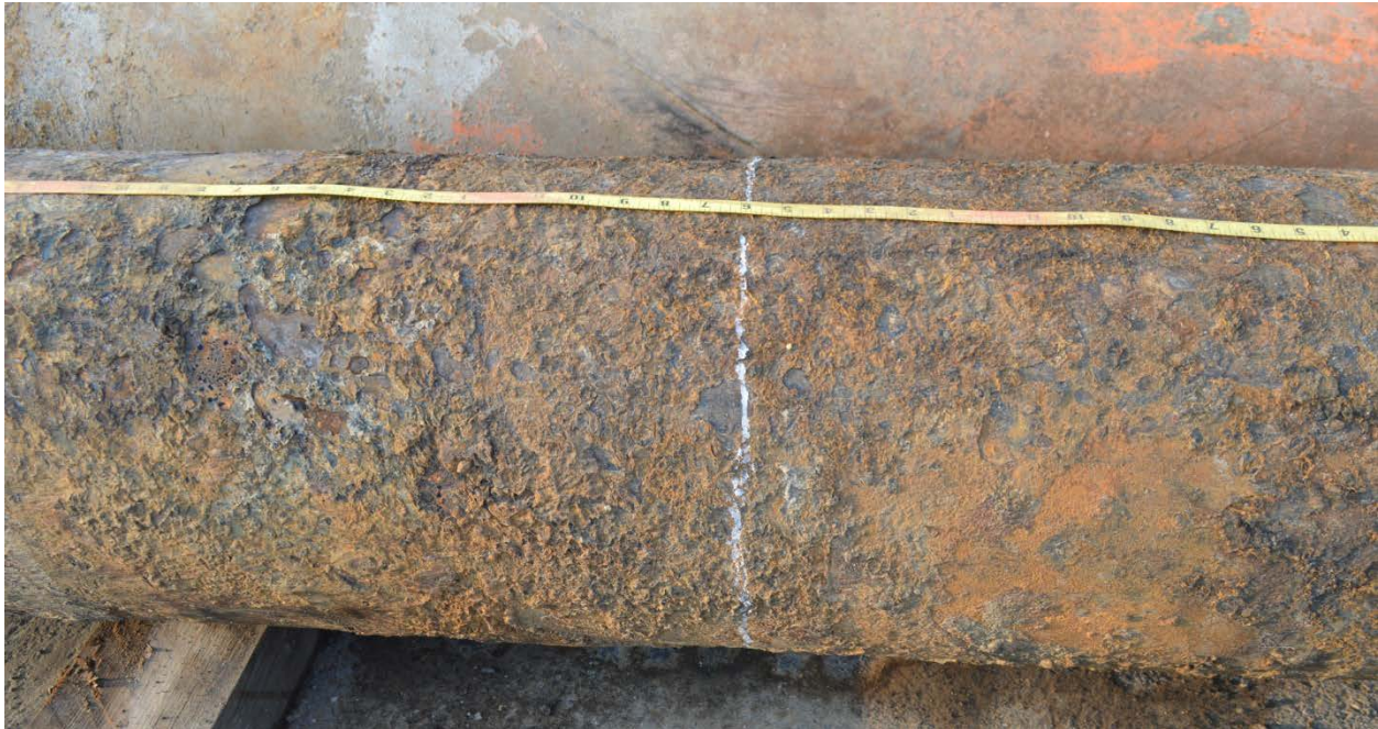
Figure 40: Close-up view of segment of exhumed CIP pile with surface corrosion. White line is location of future cut to expose pile cross-section.
