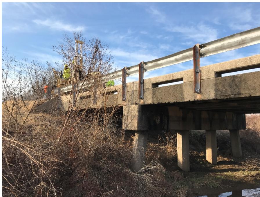
Figure 10: Photo of west end of the Route U precast pile bridge prior to replacement.
