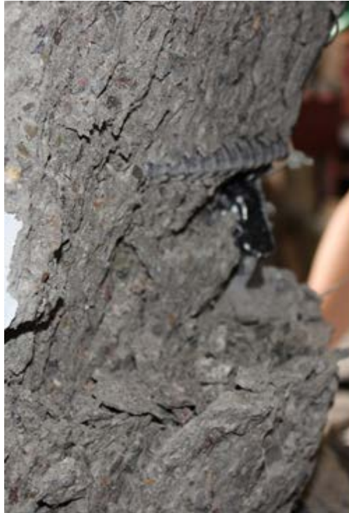
Figure 3.8 – Buckled bar #1 at south face of Specimen #1 during 2 nd cycle of -8% drift
