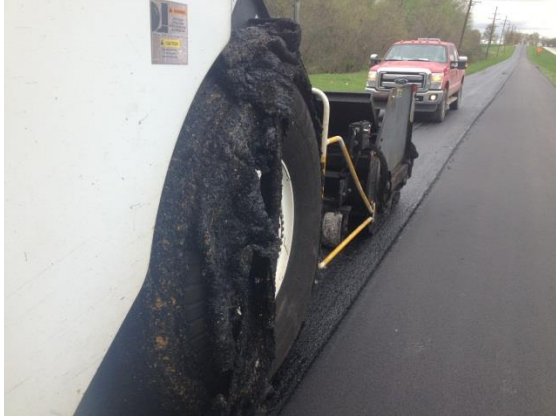
Figure 4.7 Polymer Tack Build Up (2)
