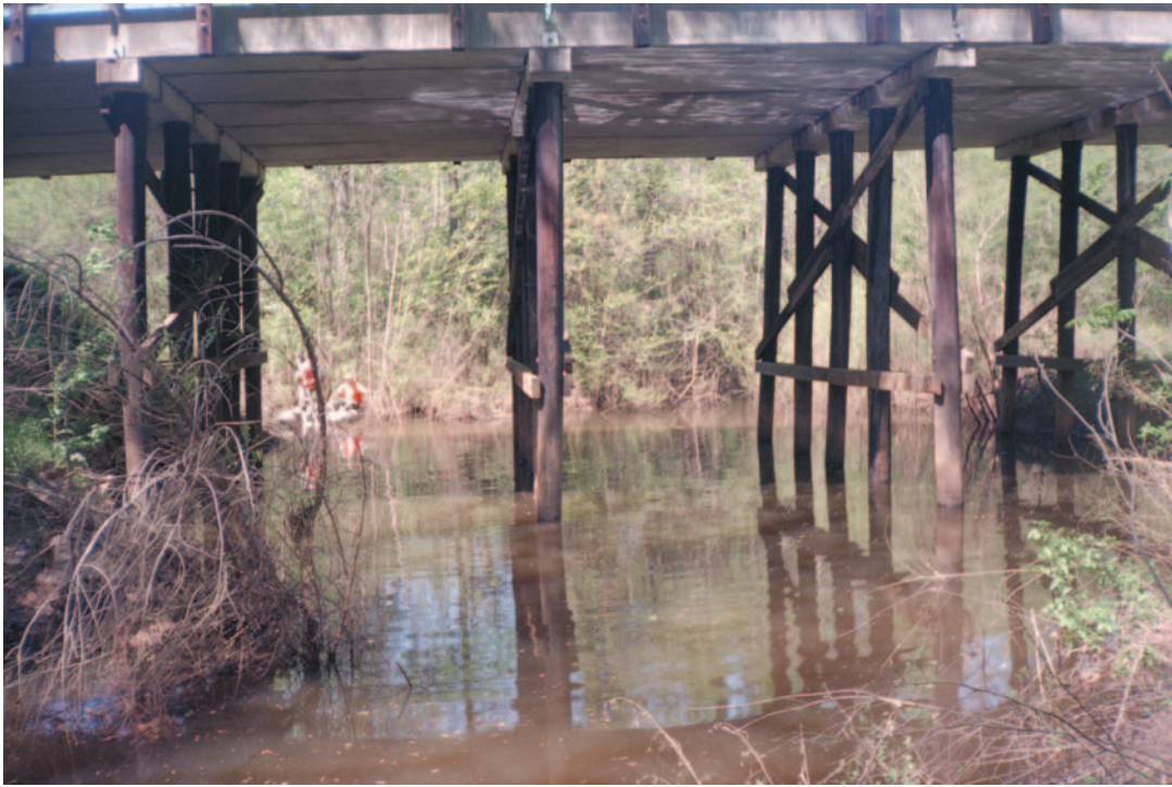
Figure 97. Right abutment-scour hole as viewed from downstream at Structure 367008100200 on Road S-81, crossing the Enoree River in Newberry County, South Carolina. The abutment-scour hole is inundated with ponded water. (Photograph by the South Carolina District, U.S. Geological Survey, April 7, 1997.)
