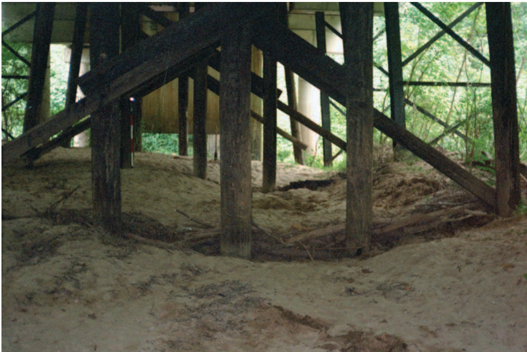
Figure 100. Example of shallow clear-water contraction scour at Structure 114000500200 on S.C. Route 5, crossing Buffalo Creek in Cherokee County, South Carolina. (Photograph by the South Carolina District, U.S. Geological Survey, October 7, 1996.)
