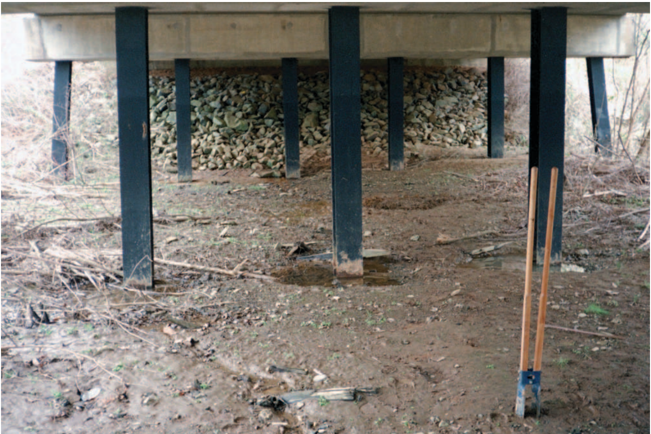
Figure 20. Steel H-pile bent at Structure 467072100100 on Road S-721, crossing Taylors Creek in York County, South Carolina. (Photograph by the South Carolina District, U.S. Geological Survey, January 29, 1997.)
