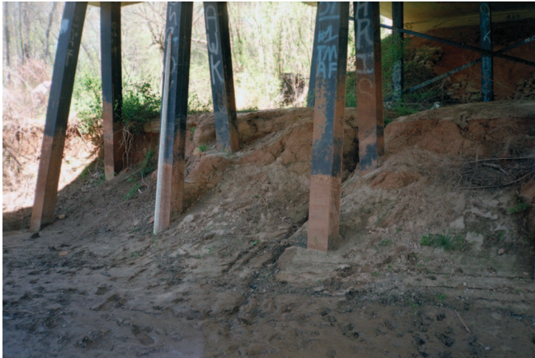
Figure 105. Erosion of bed material from around piles caused by bank widening from the August 1995 flood at Structure 307026300100 on Road S-263, crossing the Enoree River in Laurens County, South Carolina. (Photograph by the South Carolina District, U.S. Geological Survey, April 1, 1997.)
