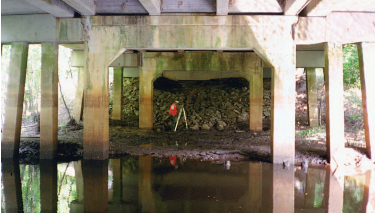
Figure 25. Composite bent at Structure 262050103200 on U.S. Route 501, crossing the Waccamaw River in Horry County, South Carolina. (Photograph by the South Carolina District, U.S. Geological Survey, June 13, 2000.)
