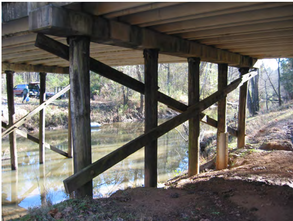
Figure 13. Timber pile bent at structure 337008500100 on Road S-85, crossing Hard Labor Creek in McCormick County, South Carolina. (Photograph by the U.S. Geological Survey, South Carolina Water Science Center, December 4, 2006.)
