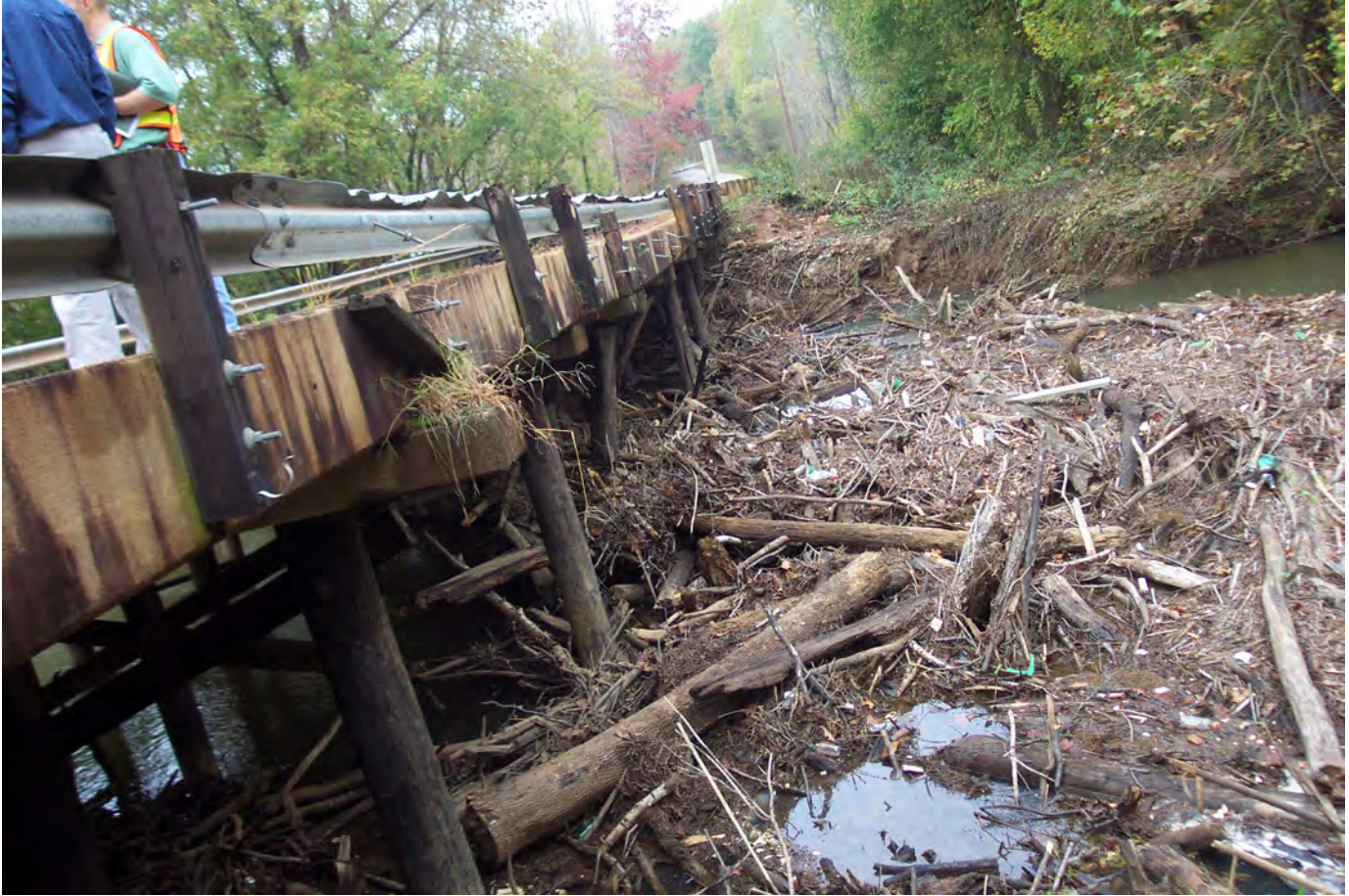
Figure 80. Example of debris accumulation that can increase scour potential at structure 427095600100 on Road S-956 crossing the North Pacolet River in Spartanburg County, South Carolina (October 9, 2004). (Photograph provided by the South Carolina Department of Transportation.)
