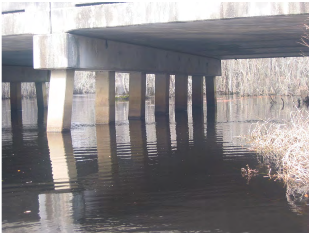
Figure 15. Square concrete pile bent at structure 174000900200 on S.C. Route 9, crossing the Little Pee Dee River in Dillon County, South Carolina. (Photograph by the U.S. Geological Survey, South Carolina Water Science Center, March 9, 2006.)
