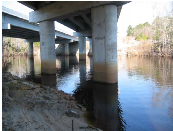
Figure 17. Pier supported on pile groups at structure 264002220100 on S.C. Route 22, crossing the Waccamaw River in Horry County, South Carolina. (Photograph by the U.S. Geological Survey, South Carolina Water Science Center, February 27, 2007.)
