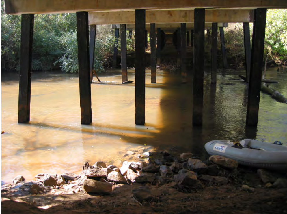
Figure 14. Steel H-pile bent at structure 237006800100 on Road S-68, crossing the Reedy River in Greenville County, South Carolina. (Photograph by the U.S. Geological Survey, South Carolina Water Science Center, October 25, 2006.)
