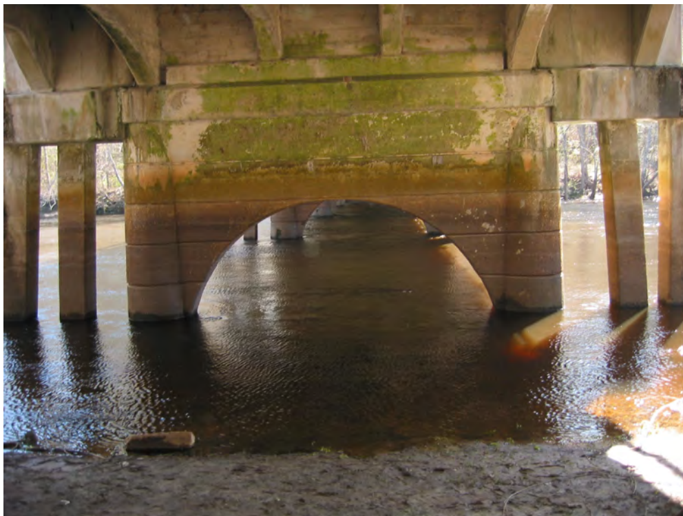
Figure 19. Composite bent at structure 182001500100 on U.S. Route 15, crossing the Edisto River in Dorchester County, South Carolina. (Photograph by the U.S. Geological Survey, South Carolina Water Science Center, March 14, 2006.)
