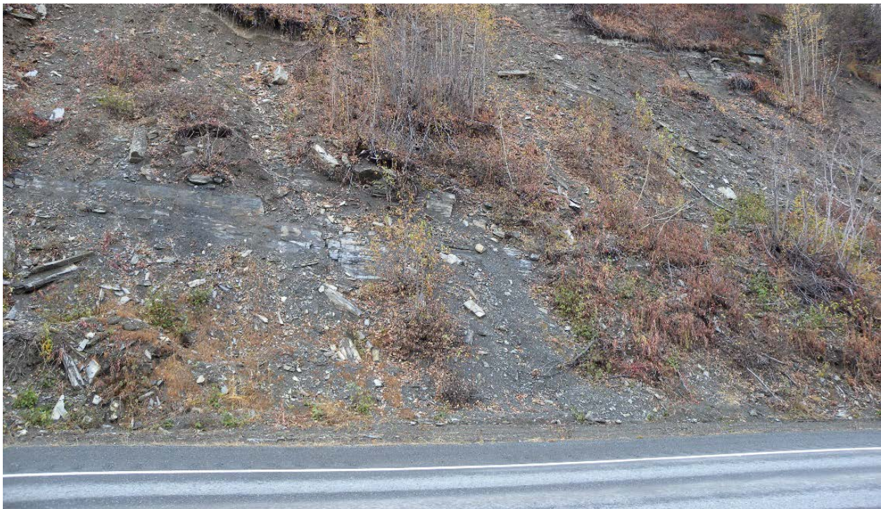
Exhibit 1. Rock slope in fair condition, South Tongass Highway. Rocks occasionally reach the road and cause a safety hazard.
