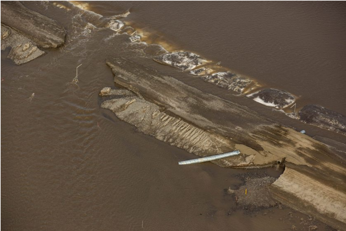
Exhibit 7. April 2015 washout of the Dalton Highway
