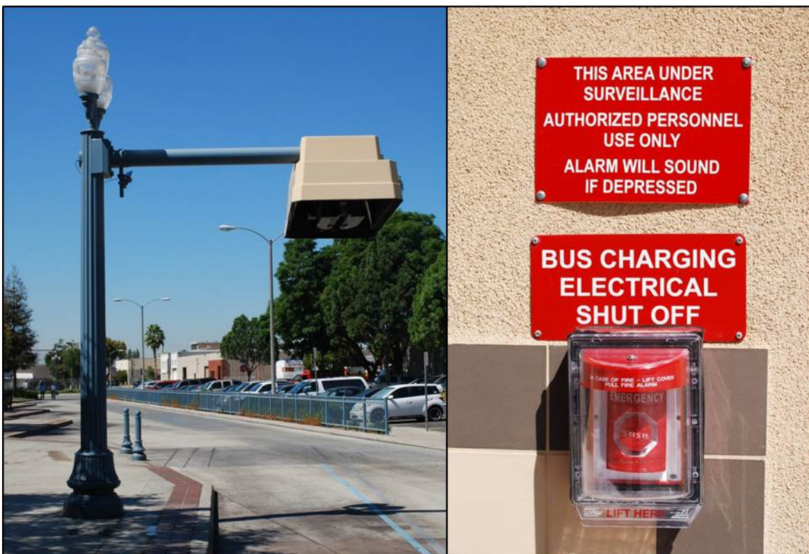
Figure 7. A charging head (left) and an emergency shut-off control (right) at the PTC
