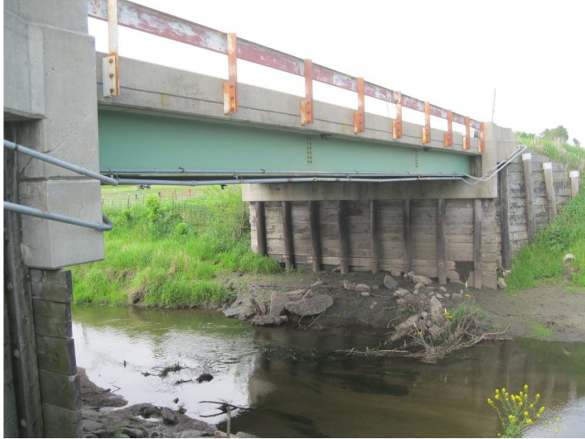
Figure 1. Instrumented bridge located on Story County Road E-18
