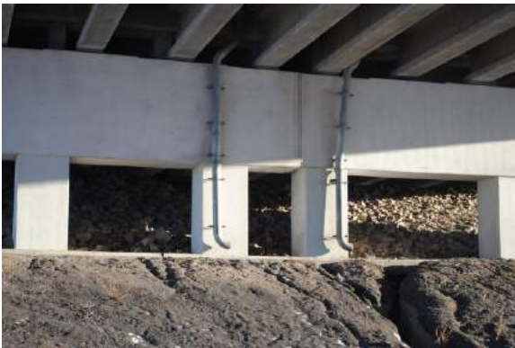
c) Down chute piping, inside lanes.
