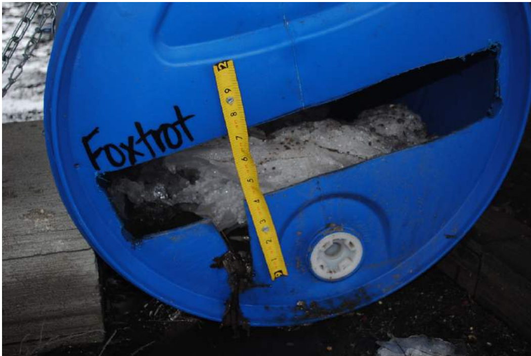
b) April 3, 2014, Location F, debris and ice damming flow through V-notch weir.
