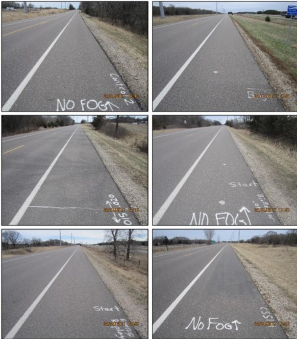
Figure 5.22 Year Three dry-condition photos clockwise from upper left: WB Control, Jointbond®, Biorestor® 0.015, CSS-1h, RePlay™, and Biorestor® 0.020.
