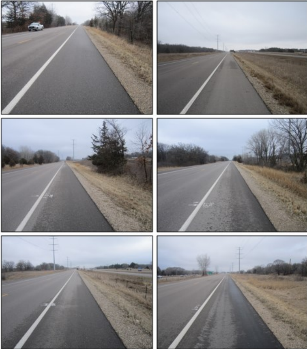
Figure 5.20 Year Two wet-condition photos clockwise from upper left: WB Control, Jointbond®, Biorestor® 0.015, CSS-1h, RePlay™, and Biorestor® 0.020.
