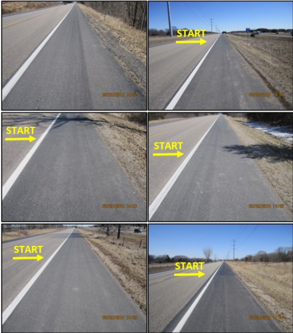
Figure 5.23 Year Four following routine fog seal, condition photos clockwise from upper left: WB Control, Jointbond®, Biorestor® 0.015, CSS-1h, RePlay™, and Biorestor® 0.020.
