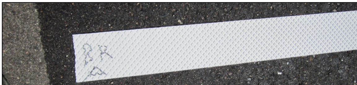
Figure 3.9 Close-up of transverse striping.
