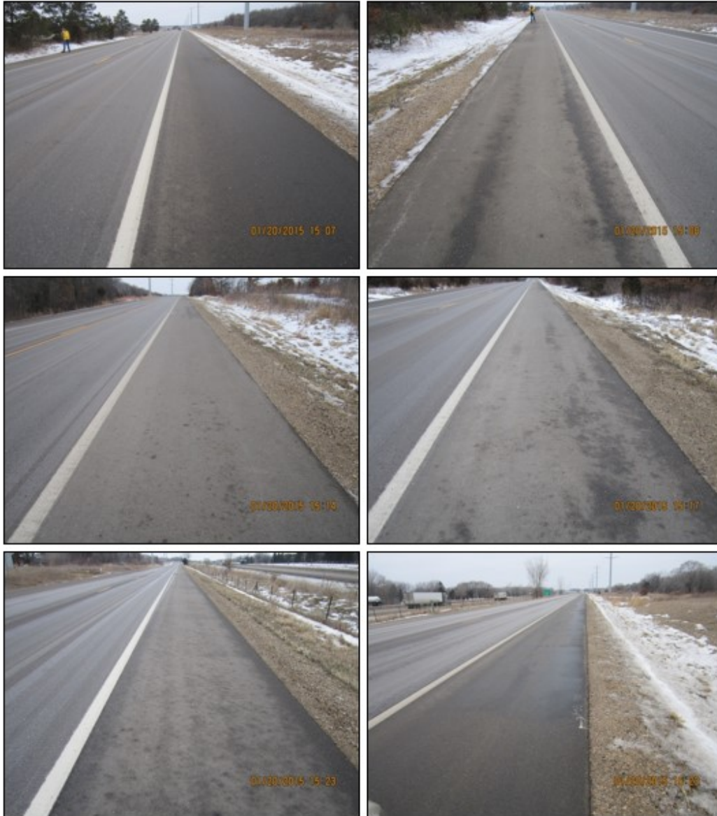
Figure 5.19 Year One wet-condition photos clockwise from upper left: WB Control, Jointbond®, Biorestor® 0.015, CSS-1h, RePlay™, and Biorestor® 0.020.
