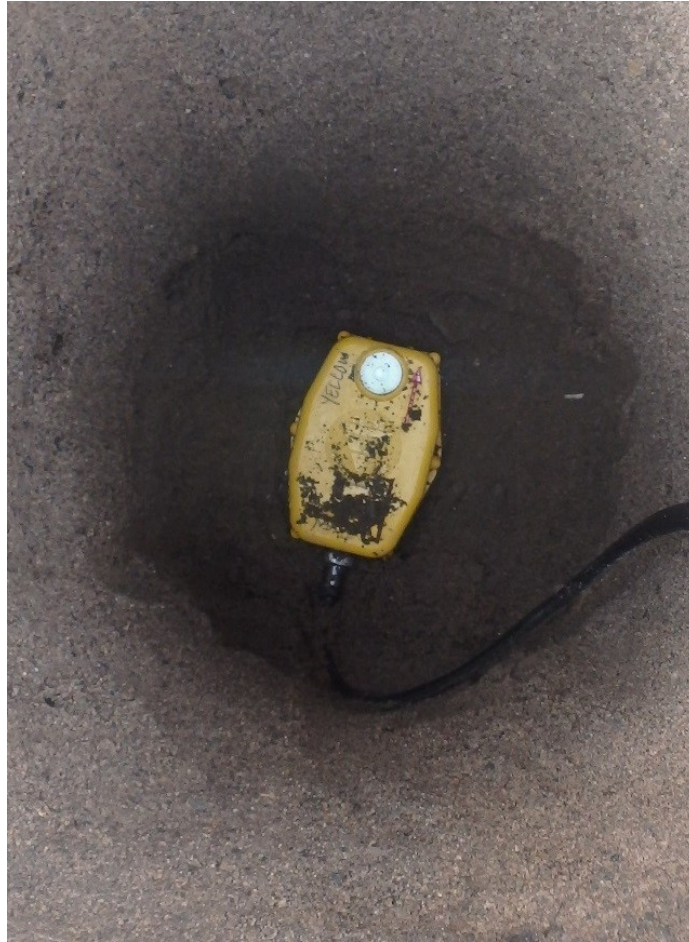
Figure 10.7 Geophone installed in a MnROAD section.
