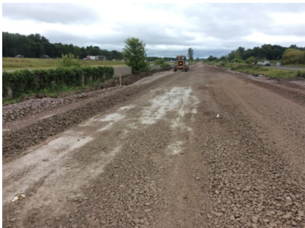
Figure 7.8 Comparison of large stone subbase condition: 9-inch thick Cell 128 (foreground) and 18-inch thick Cell 227 (background).
