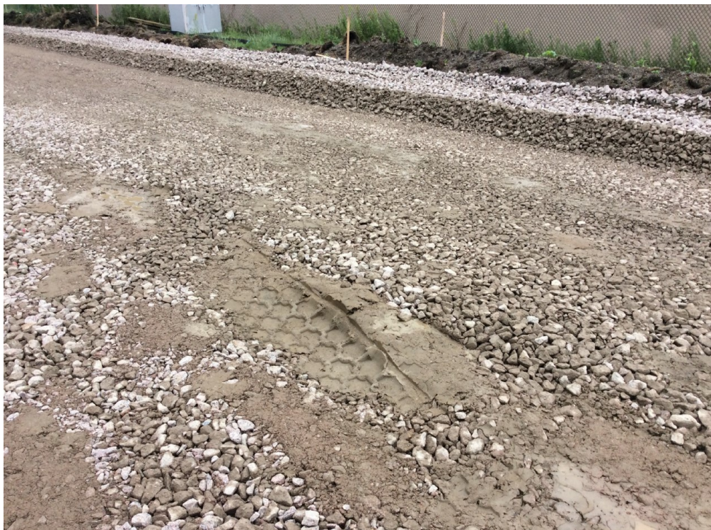
Figure 7.7 Condition of 9-inch deep large stone subbase section after first construction iteration.
