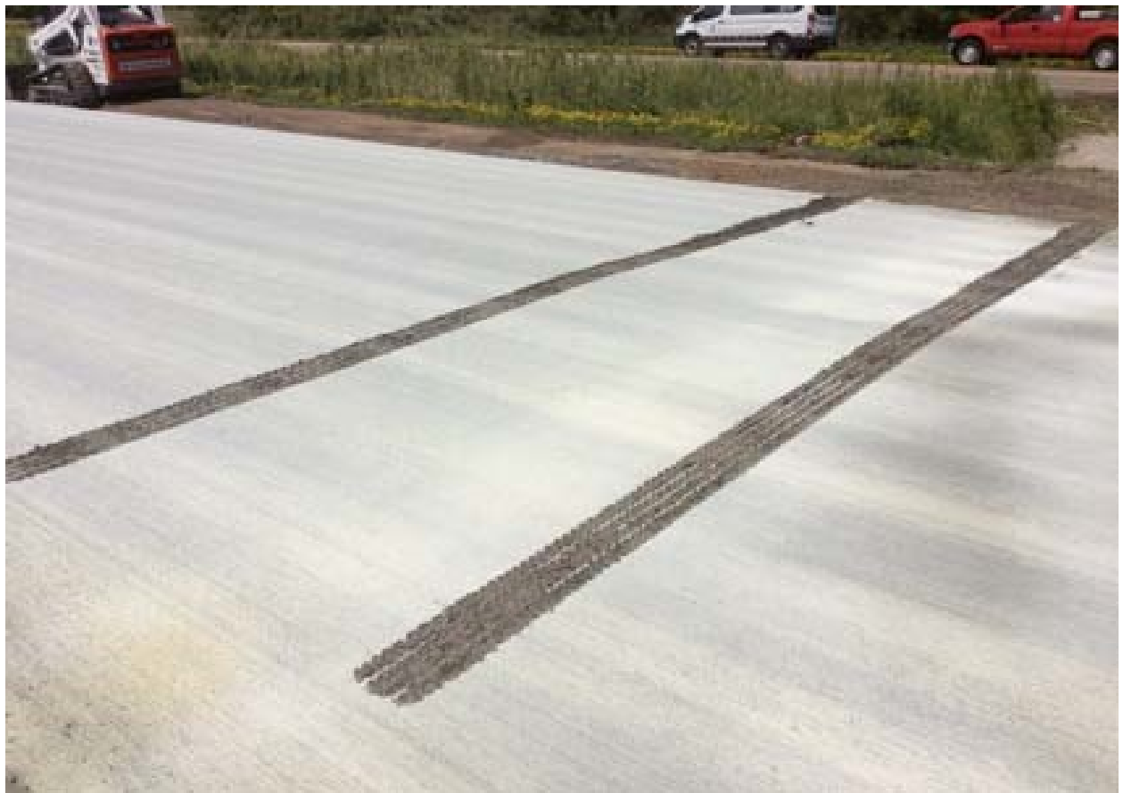
Figure 5.6 Rut depth ranged from 0.25 inch in the outside lane to 1.5 inches at the edge of inside lane.
