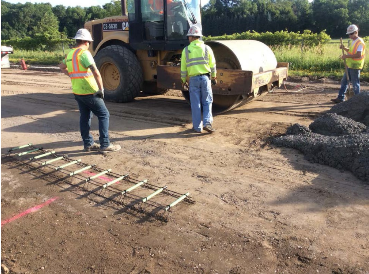
Figure 6.4 Contractor shaping aggregate base in front of paver with drum roller, Cell 238.
