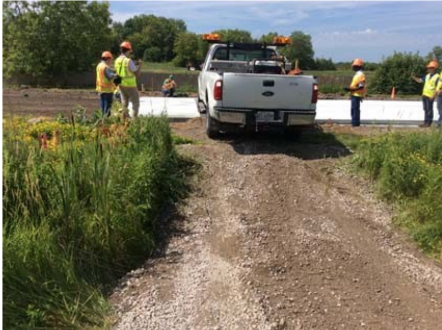
Figure 5.5 Preparation in the second hour for application of rut on sub-Cell 624 plastic concrete.
