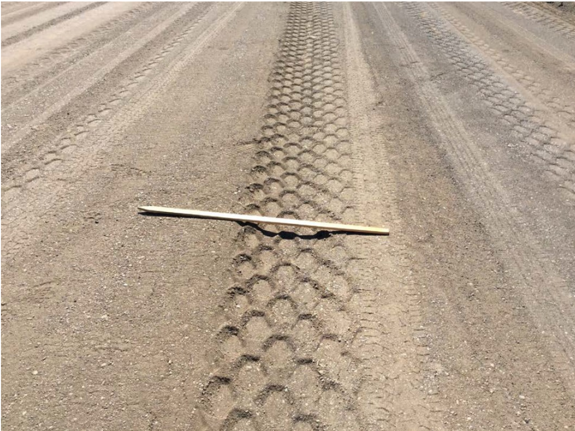
Figure 6.3 Rut in Cell 238 aggregate base due to passage of intelligent compaction steel drum roller.
