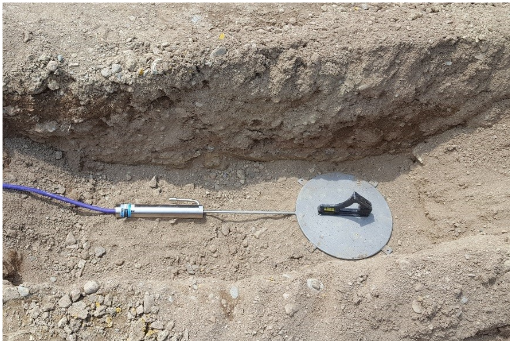
Figure 10.6 Dynamic pressure cells (PG) installed in a MnROAD section.
