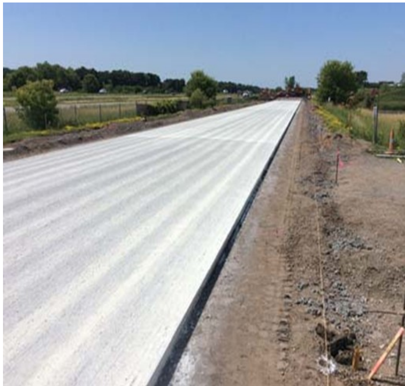
Figure 5.4 Panoramic view of Cells 124 to 624 pavement after placement and application of curing compound.
