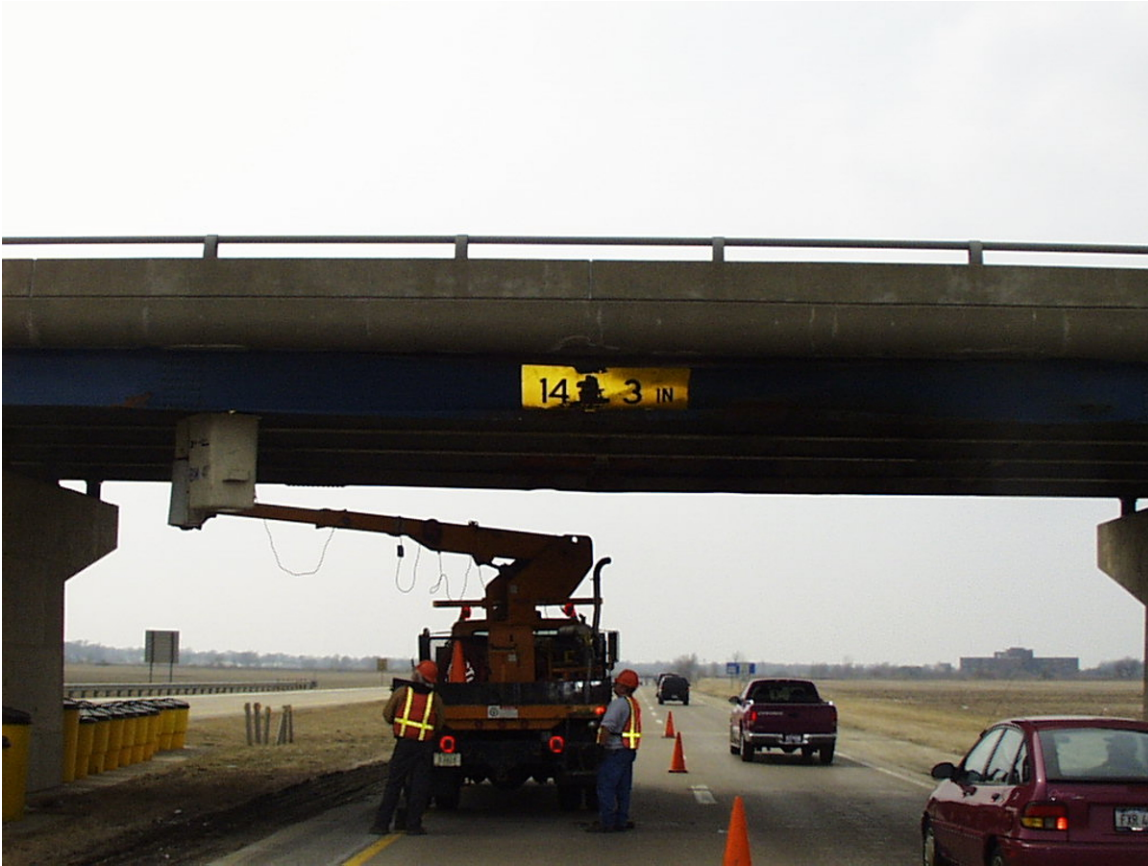
Photo of IDOT maintenance crews assessing damage to a struck overpass bridge on U.S. 34. Photo courtesy of IDOT.
