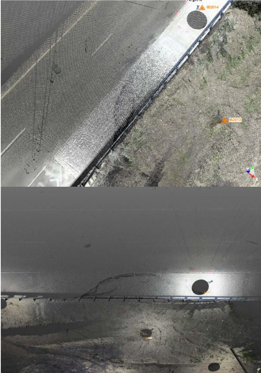
Figure 11. Route 251 Slope Failure – Shoulder Erosion, laser scanner generated point clouds with images superimposed.
