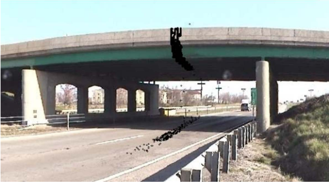
Damaged bridge girder with a 4-ft slice of a point cloud scan. Source: FHWA-ICT-10-068 Report
