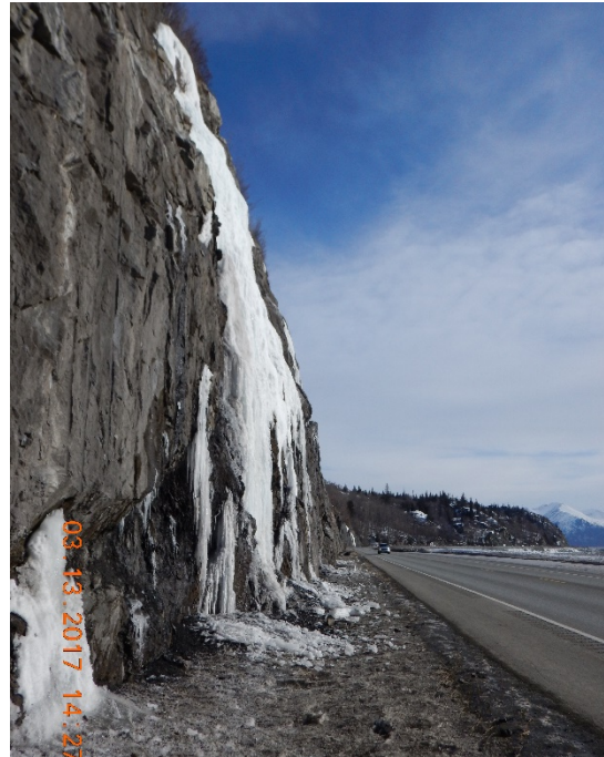
Figure 24 – Ice conditions along ditch near MP 113.2 on 13 March 2017 (Photo by Scarptec, Inc.)
