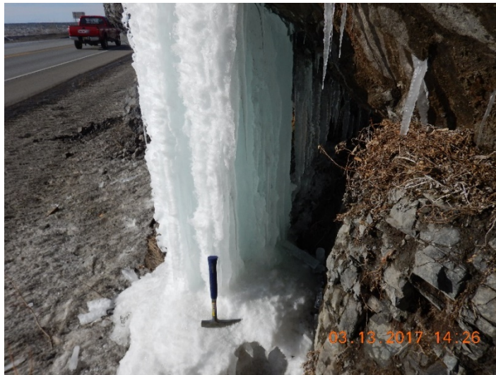
Figure 5 – Partial ice column direct bearing near MP 113.2 NB on the Seward Highway (Photo by Scarptec, Inc.)
