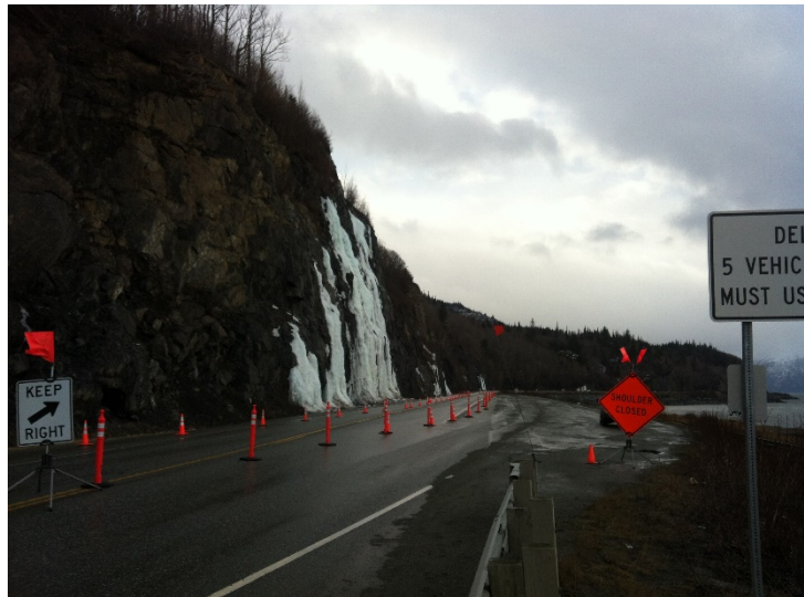
Figure 18 – Traffic pattern modification and detour at MP 113.2 area (Photo by Alaska DOT&PF)
