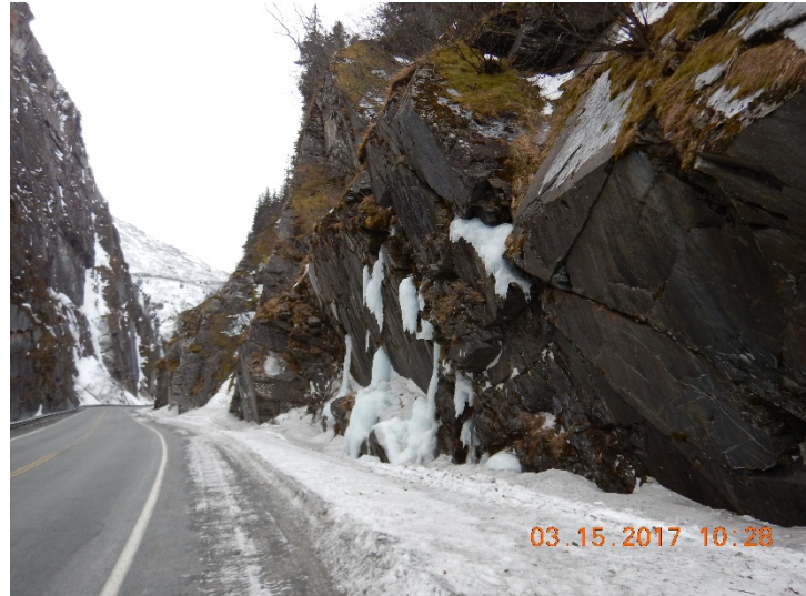
Figure 33 – Limited ice development near MP 13.9 SB along Richardson Highway on 15 March 2017 (Photo by Scarptec, Inc.)
