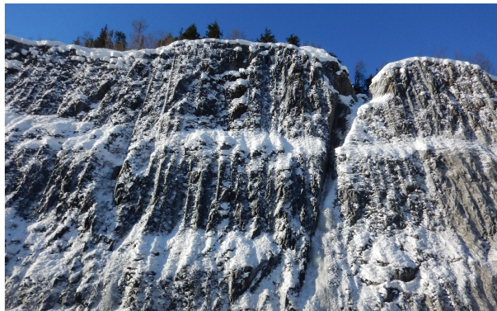
Figure 28 – Minor ice in fracture near MP 58.1 NB along Seward Highway (Photo by Scarptec, Inc.)
