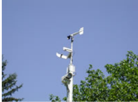
Figure 16 – RWIS onsite instrumentation for remote data transmission (Photo by Alaska DOT&PF)
