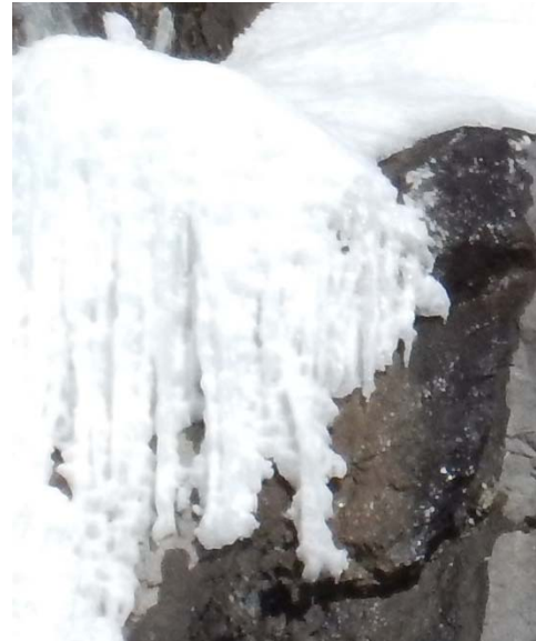
Figure 15 – Interface retraction seen at MP 113.2 NB on the Seward Highway in March 2017 (Photo by Scarptec, Inc.)
