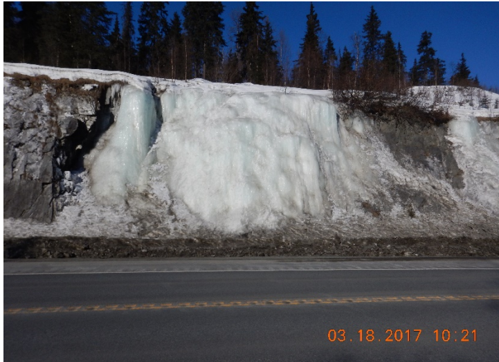
Figure 27 – Ice slab conditions near MP 57.9 NB along Seward Highway (Photo by Scarptec, Inc.)
