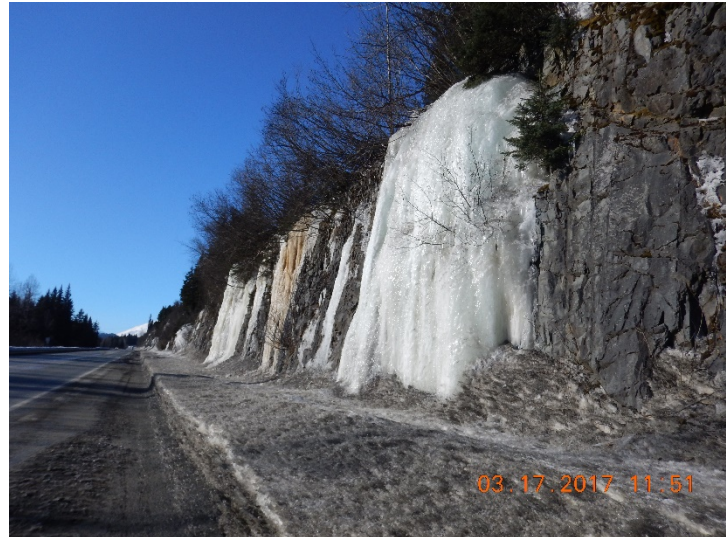
Figure 26 – Ice slab conditions adjacent to MP 74.8 SB along Seward Highway (Photo by Scarptec, Inc.)
