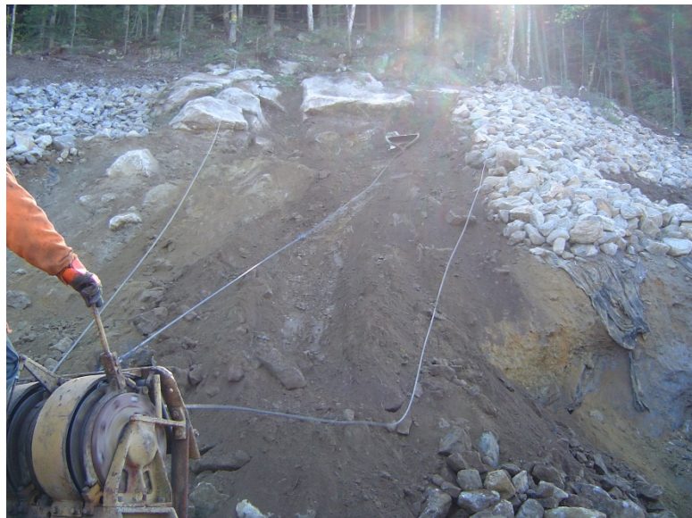
Figure 17 – Picture of “slusher” scraping the slope of loose debris (Photo by Ameritech Slope Constructors, Inc.)
