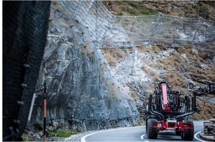
Figure 19 – Slotted icefall netting & upslope flexible barrier in Austria (Photo by Trumer, Ltd.)
