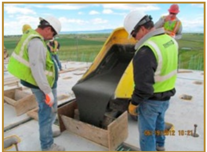
Figure 1: Field-cast joint being filled with proprietary UHPC on a previous MDT Project
