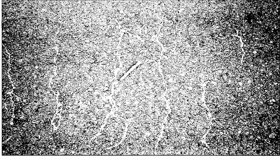
Figure A-1. Typical fatigue cracking pattern at WestTrack.
