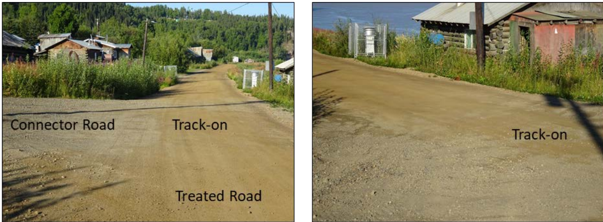
Figure 17. Evidence of track-on
