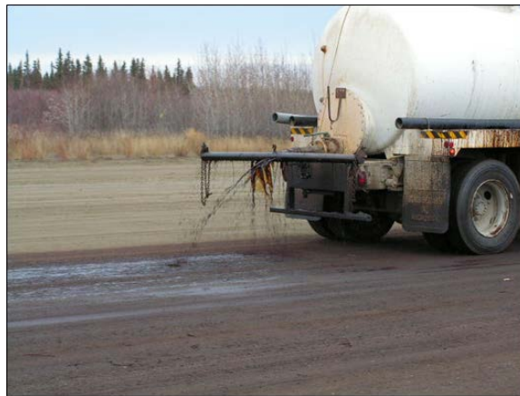
Figure 11. Incorrect application of synthetic fluid with a water truck (photo courtesy of ADOT&PF)
