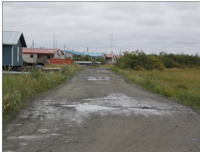
Figure 7. Improperly graded road resulting in poor drainage off of the road surface
