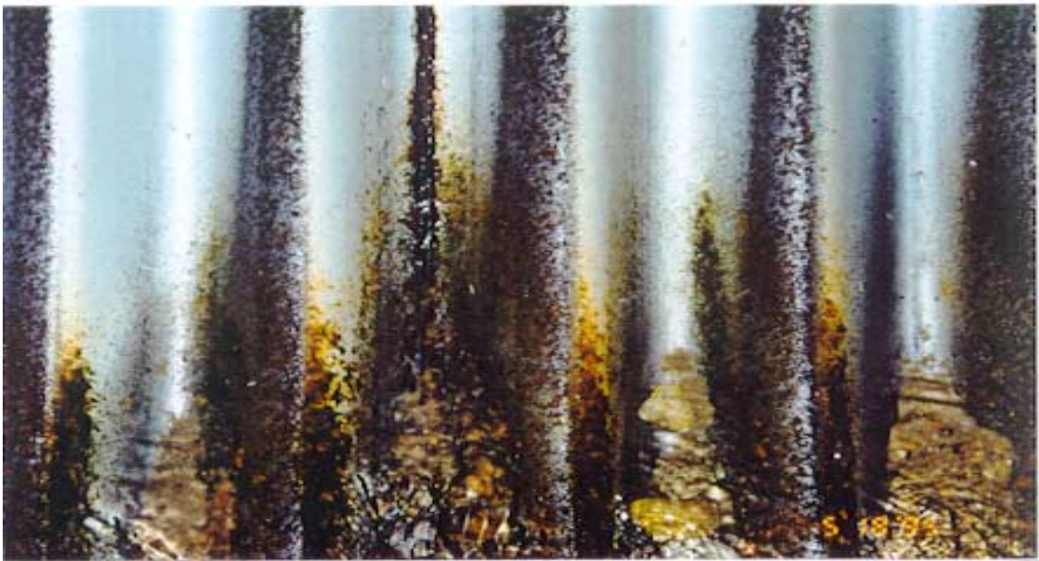
Figure 5. Close-up of 310.0 (flow is from left of photo to right). Note: Wear and corrosion predominate on upstream side of corrugation.
