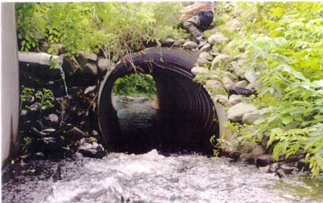
Figure 7. Culvert at Dexter, Maine, experiencing high-velocity flow.
