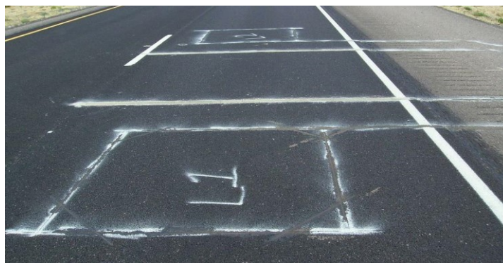
Figure 5. Photo. Double threshold WIM system setup with piezoquartz sensors. (33)
