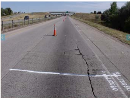
Figure 25. Longitudinal cracking near the shoulder in Colorado-0217 section (September 20, 2011).
