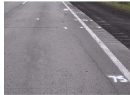
Figure 30. Longitudinal cracking near the shoulder in Washington-0206 section (May 23, 2013).
