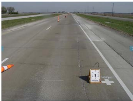
Figure 29. Longitudinal cracking near the shoulder in Ohio-0206 section (September 12, 2006).
