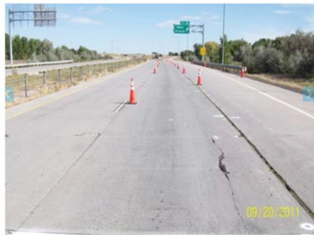
Figure 26. Longitudinal cracking near the shoulder in Colorado-0218 section (September 20, 2011).
