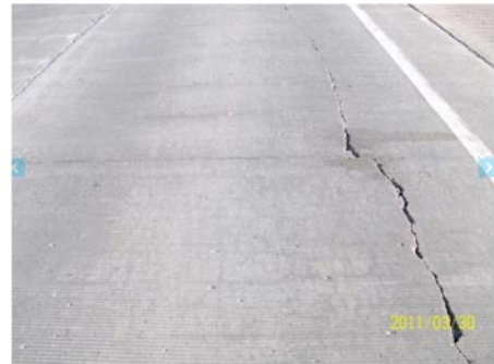
Figure 28. Longitudinal cracking near the shoulder in Iowa-0217 section (March 30, 2011).
