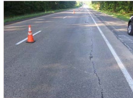
Figure 24. Longitudinal cracking near the shoulder in Arkansas-0217 section (December 4, 2012).
