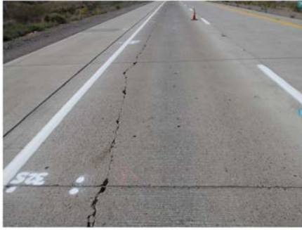
Figure 21. Longitudinal cracking near the shoulder in Arizona-0213 section (February 16, 2011).
