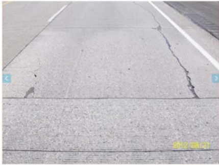
Figure 27. Longitudinal cracking near the shoulder in North Dakota-0217 section (August 21, 2012).
