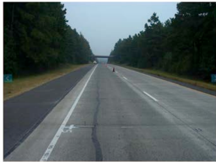
Figure 23. Longitudinal cracking near the shoulder in Arkansas-0213 section (May 24, 2007).
