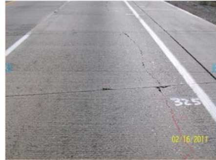
Figure 22. Longitudinal cracking near the shoulder in Arizona-0262 section (February 16, 2011).
