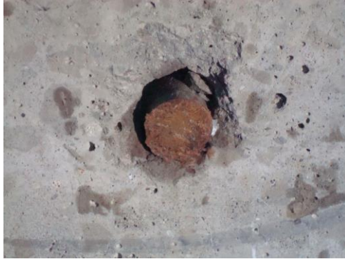
Figure 17. Poor anchoring of dowel into hole that resulted in faulting of the transverse FDR joint. (Photo Courtesy of Mark Snyder)
