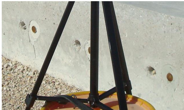
Figure 18. Use of grout retention disks provides good coverage. (Photo Courtesy of Mark Snyder)
