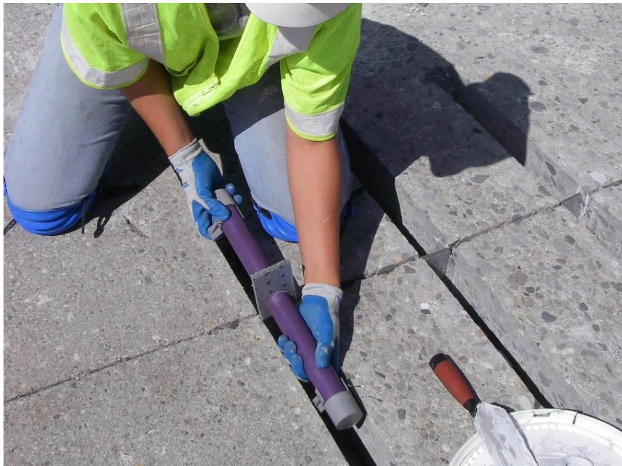
Figure 8. Inserting dowel bar assembly into slot. (Photo Courtesy of Jeff Uhlmeier, WSDOT)
