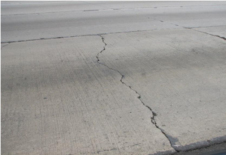
Figure 24. Midpanel cracking on an RSC slab on I-5 in Los Angeles County.
