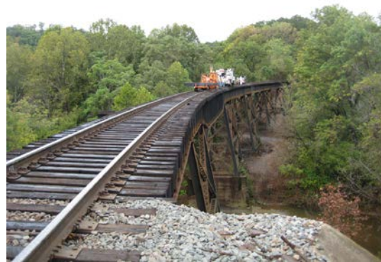
Figure 1. Track Crew Installing Rail Fasteners on the Test Bridge at NS' Eastern Mega Site
