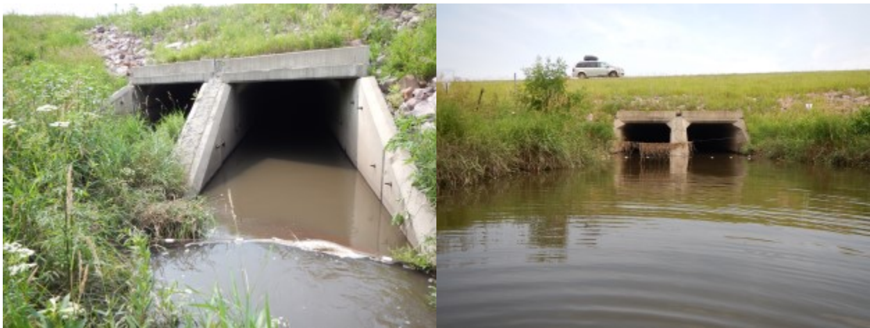
Figure 2.6 Upstream view of culvert 8884 on Split Rock Tributary, Rock County, showing vegetation in left barrel (left) and downstream view of culvert 8884 showing large pool with surrounding vegetation.
