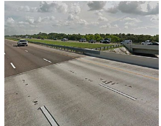
The areas where an asphalt pavement approaches or departs a concrete bridge are susceptible to specific kinds of distress.
