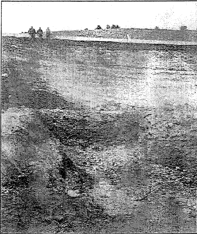
Figure 4. Excavation to expose spring and build box culvert to span spring outlet. Spring flowing 1135 liters per minute shown at lower center of photo.
