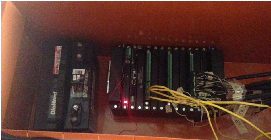
Figure 3-26 DAQ in Job Box
