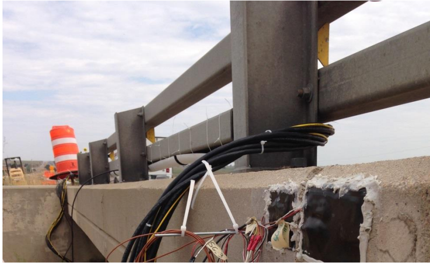
Figure 3-27 Wires Along Railing
