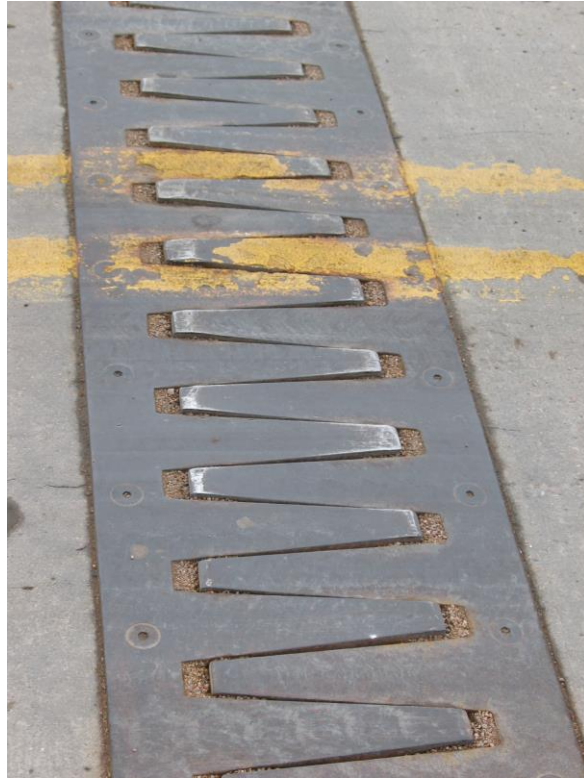
Figure 3-4. Finger Joint Clogged by Debris on B-16-FM (Photo courtesy of CDOT)
