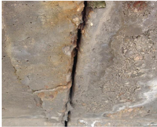
Figure 5-7 Deterioration of C-17-AT Abutments and Joints
