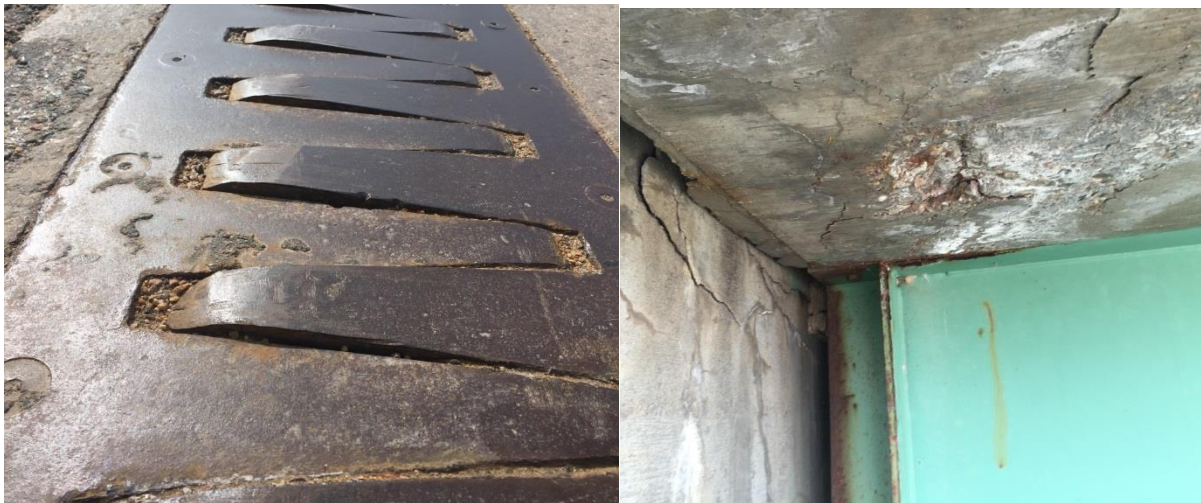
Figure 5-8 Deterioration of B-16-FM Abutments and Joints
