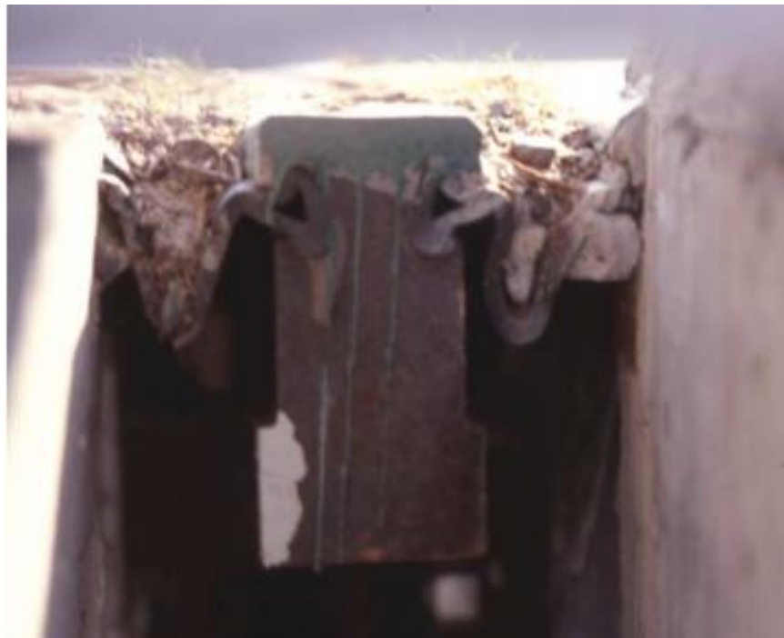
Figure 2-2. Debris in expansion joint in service for less than six months (Chen, 2008)
