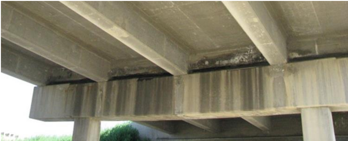
Figure 3-10 C-17-AT Underside – Corrosion & Leakage
