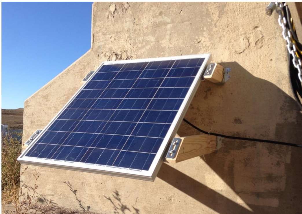
Figure 3-32 Solar Panel Attached to Abutment
