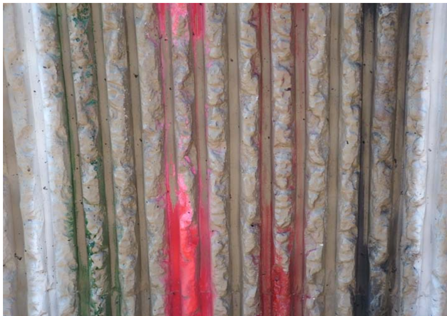
FIGURE 4.3D Close-up of Removal - Fractured Fin Facing Panel 3
