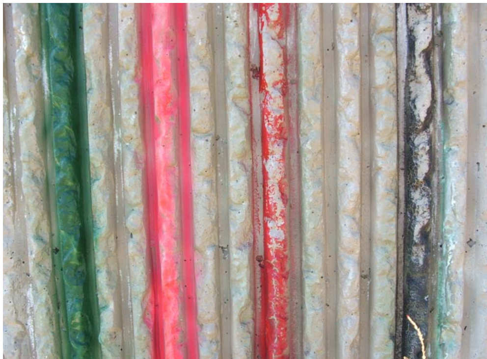
FIGURE 4.13D Close-up of Removal - Fractured Fin Facing Panel 13
