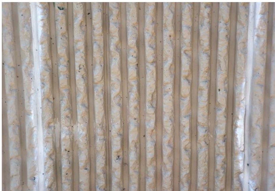
FIGURE 4.4D Close-up of Removal - Fractured Fin Facing Panel 4
