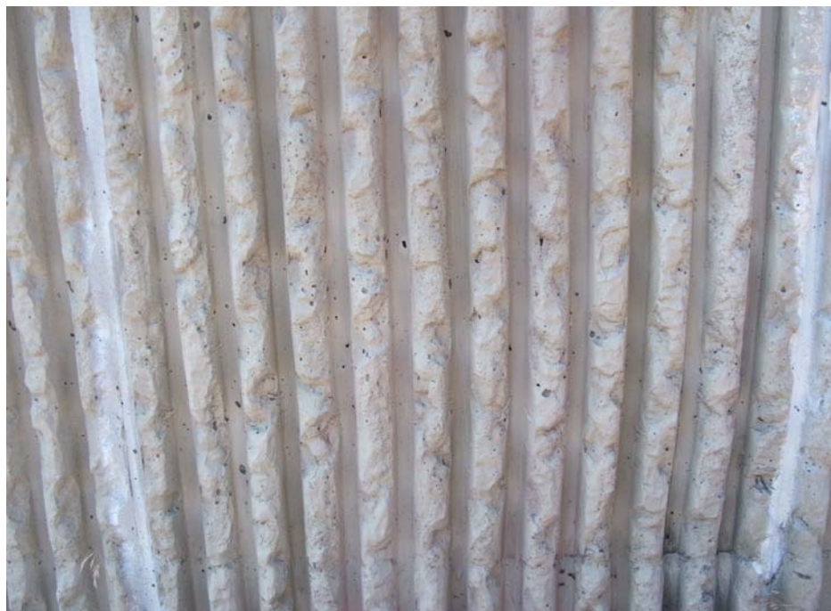
FIGURE 4.11D Close-up of Removal - Fractured Fin Facing Panel 11
