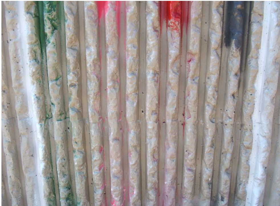
FIGURE 4.7D Close-up of Removal - Fractured Fin Facing Panel 7
