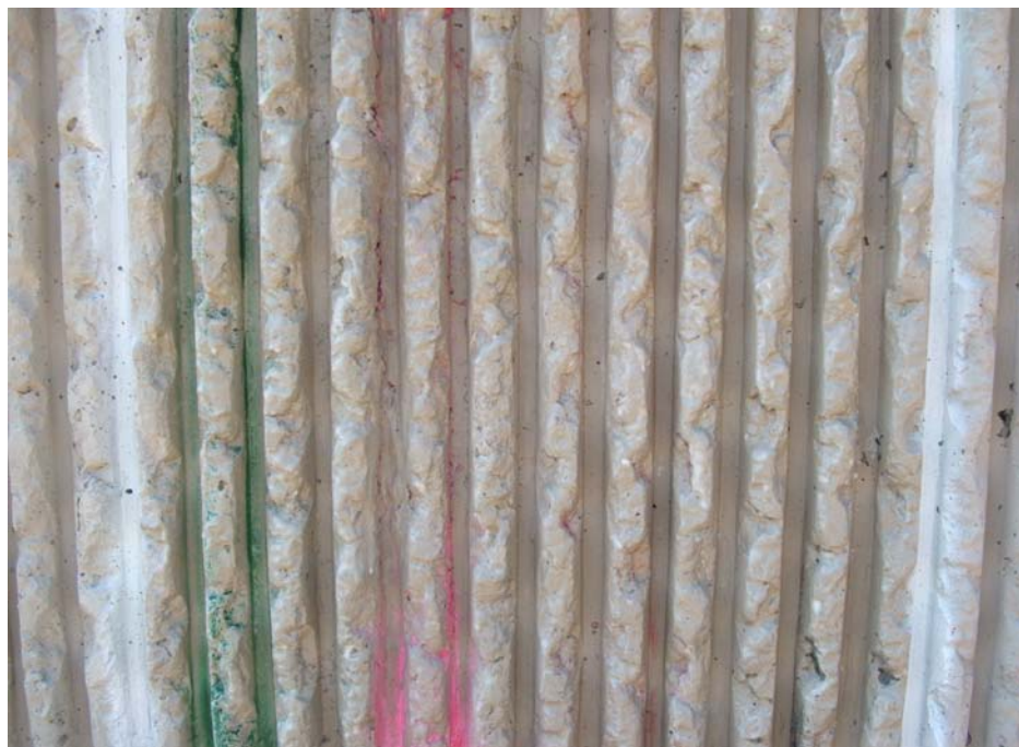
FIGURE 4.2D Close-up of Removal - Fractured Fin Facing Panel 2
