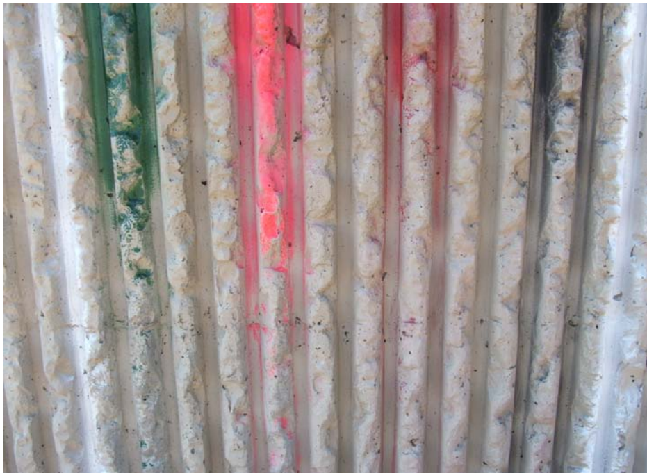
FIGURE 4.1D Close-up of Removal - Fractured Fin Facing Panel 1
