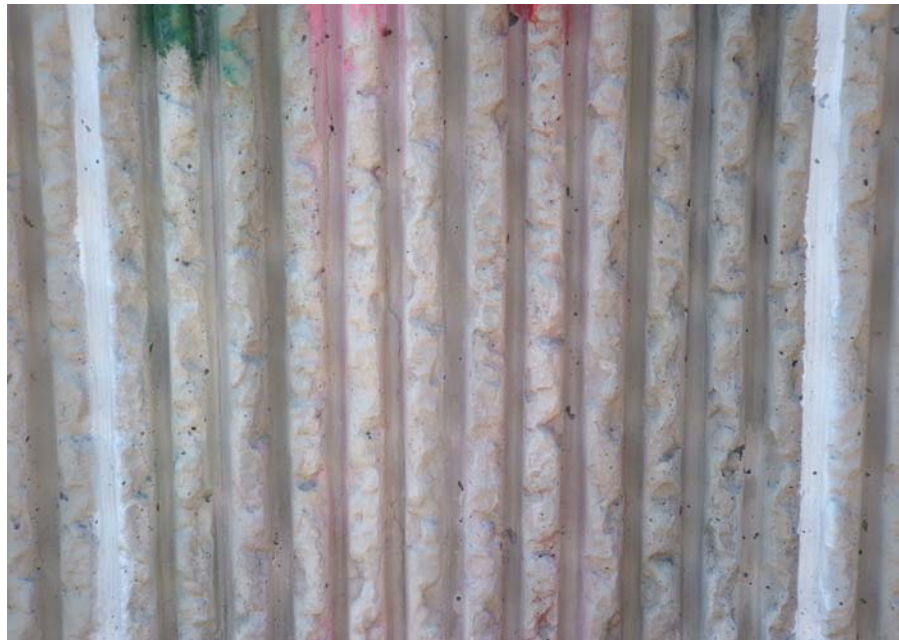
FIGURE 4.12D Close-up of Removal - Fractured Fin Facing Panel 12
