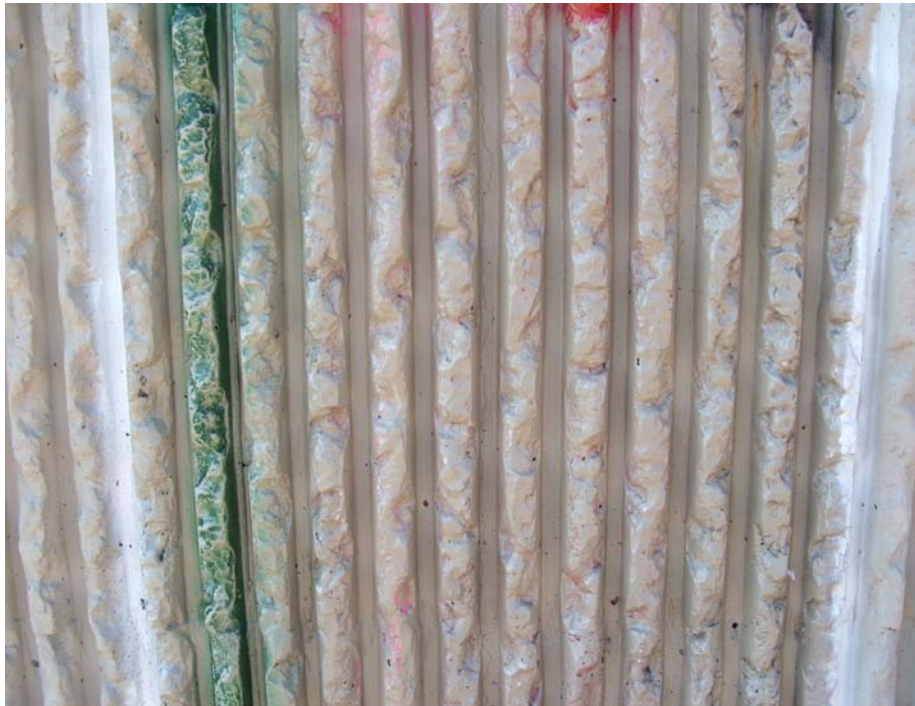
FIGURE 4.8D Close-up of Removal - Fractured Fin Facing Panel 8
