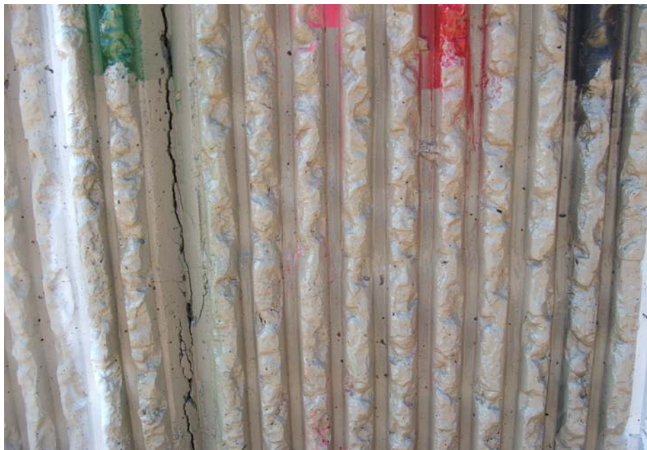
FIGURE 4.6D Close-up of Removal - Fractured Fin Facing Panel 6
