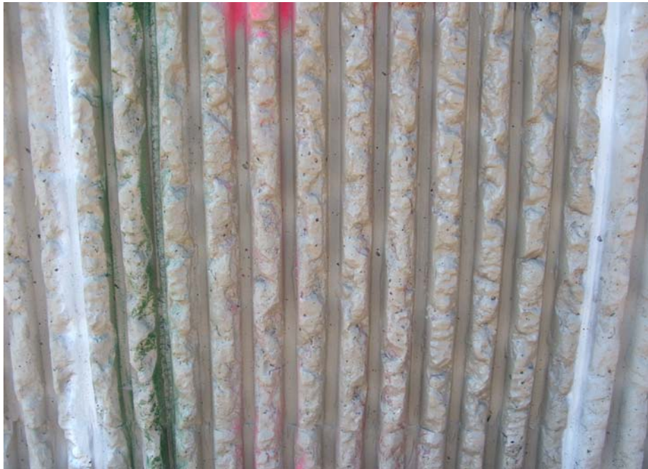
FIGURE 4.10D Close-up of Removal – Fractured Fin Facing Panel 10
