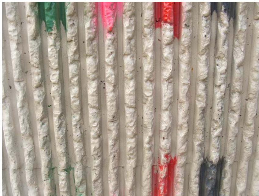
FIGURE 4.14D Close-up of Removal - Fractured Fin Facing Panel 14
