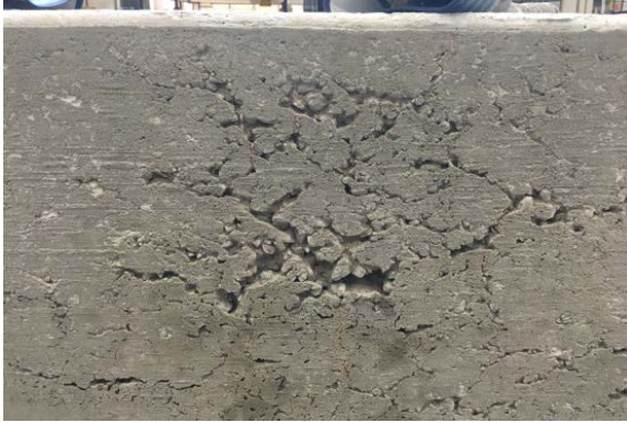
(a) Span - Honeycombing
