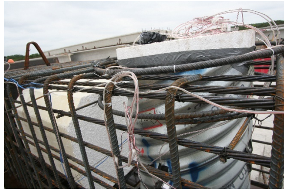
(b) PSV-28A Strain Gauged Mild Steel Reinforcement, Mild Steel Hoop, and Corrugated Steel Pipe
