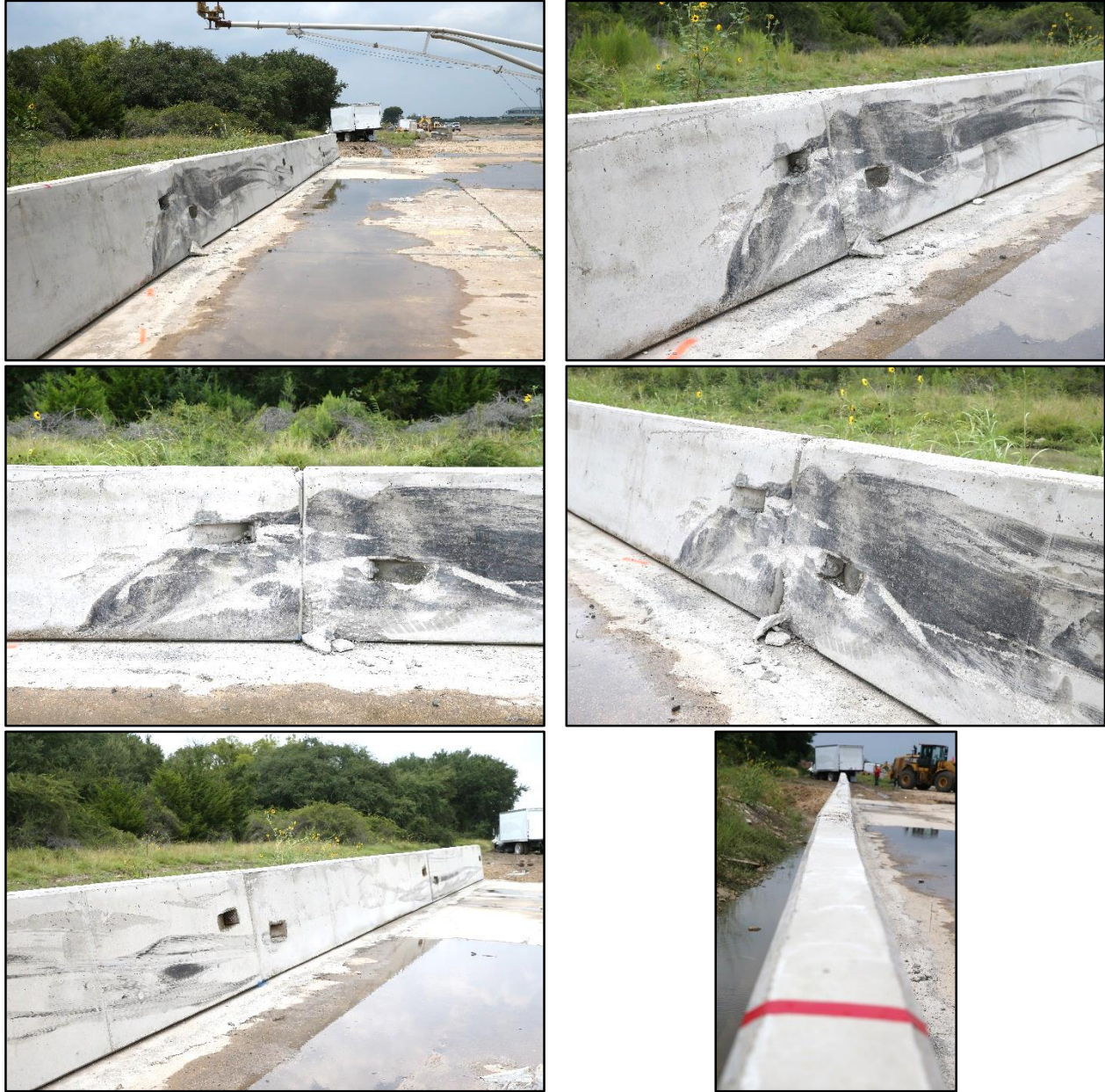
Figure 6.3. Restrained Safety Shape Concrete Barriers on Concrete Deck after Test No. 490027-2-1.
