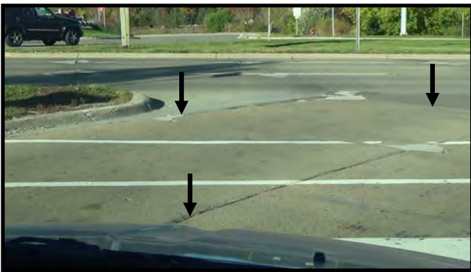
End of the HFS and Surface Spalling
