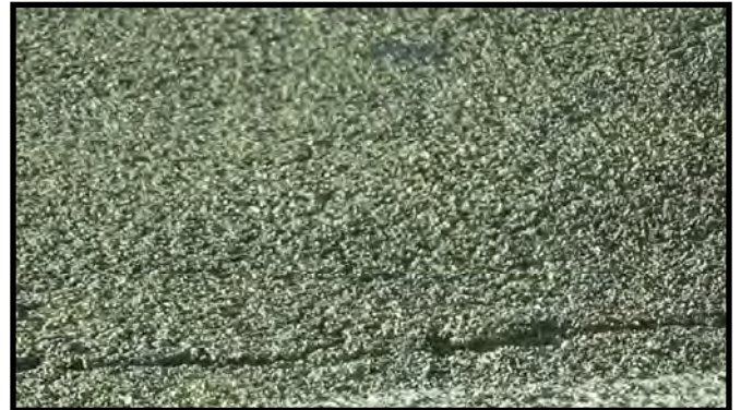
Close Up of the Installed HFS
