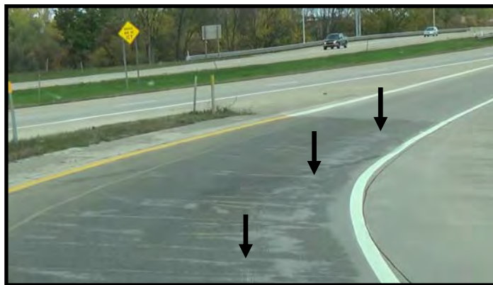
Surface Spalling at the End of the Ramp
