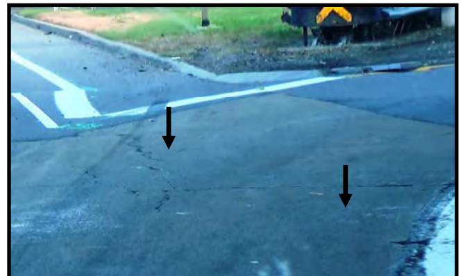
HFS Current Condition and Resurfaced Area
