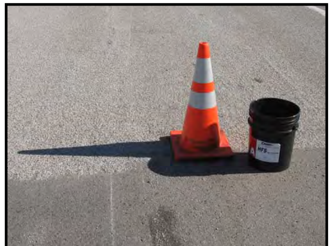
Figure 6: Loose Stone Awaiting to be Swept (Left) and Loose Stone Already Swept
