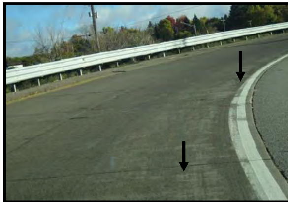
Large Amount of Surface Spalling-Right Side of Travel Lane
