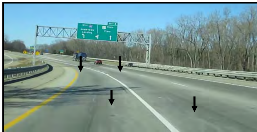
Surface Spalling Area and End of Surface
