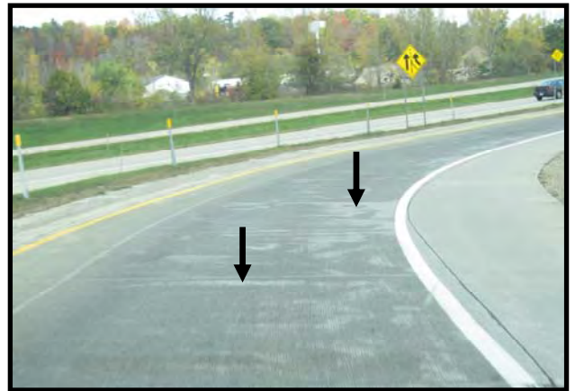
Surface Spalling in the Travel Lane
