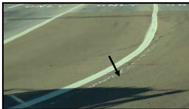
Close Up of Spalling at the Joint Lines
