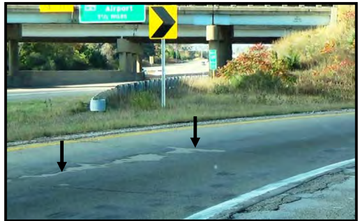
Surface Spalling in the Travel Lane
