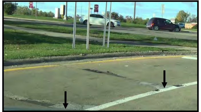
Surface Spalling at the Joint Lines
