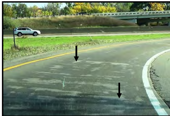
Surface Spalling at the End of Ramp
