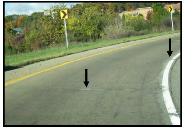
Start of the Surface Spalling at the Joint Lines
