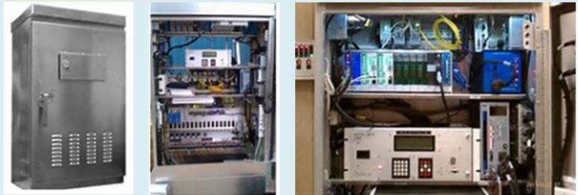
Traffic Signal Controller - cabinet and hardware
