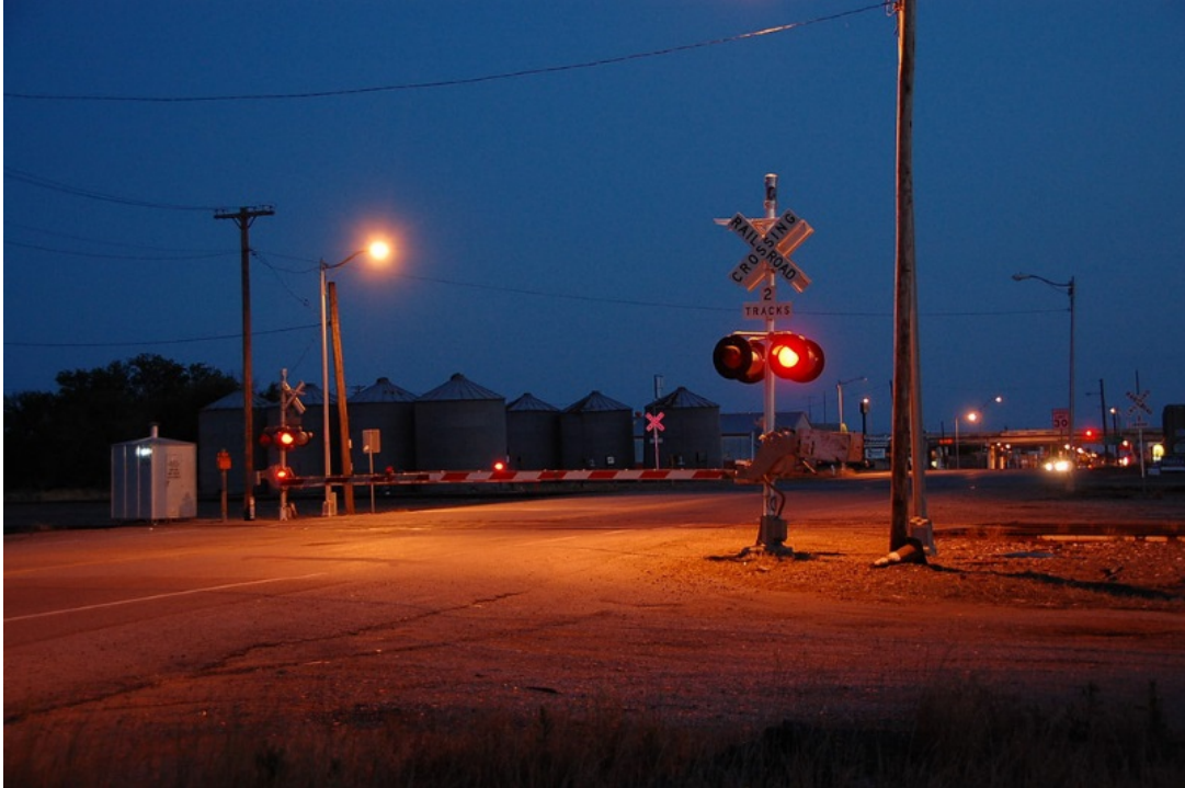
Figure 5.31: Lighting to illuminate railroad tracks and path, (N/A, N/A)
