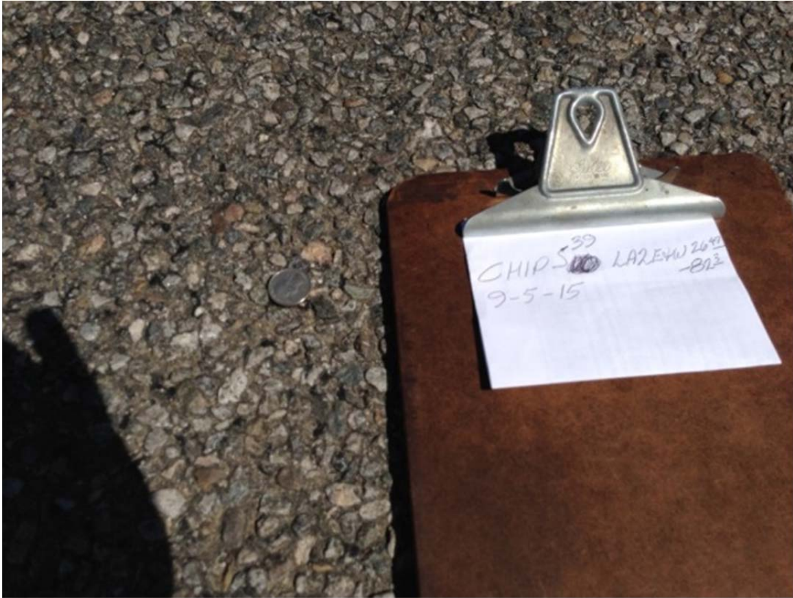
Figure 9.2: Close-up photo of pavement on LA-2.
