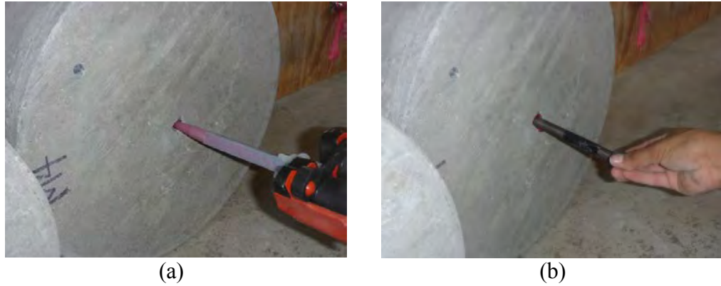
Figure 4.7: (a) Delivery of adhesive into horizontally drilled hole; (b) horizontal anchor installation
