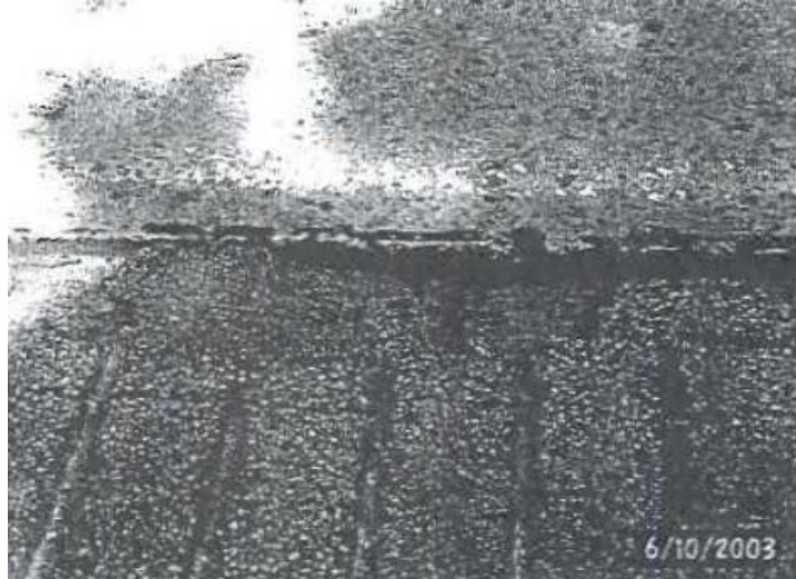
FIGURE 3.42: Example of shoulder joint distress (GDOT 2003)
