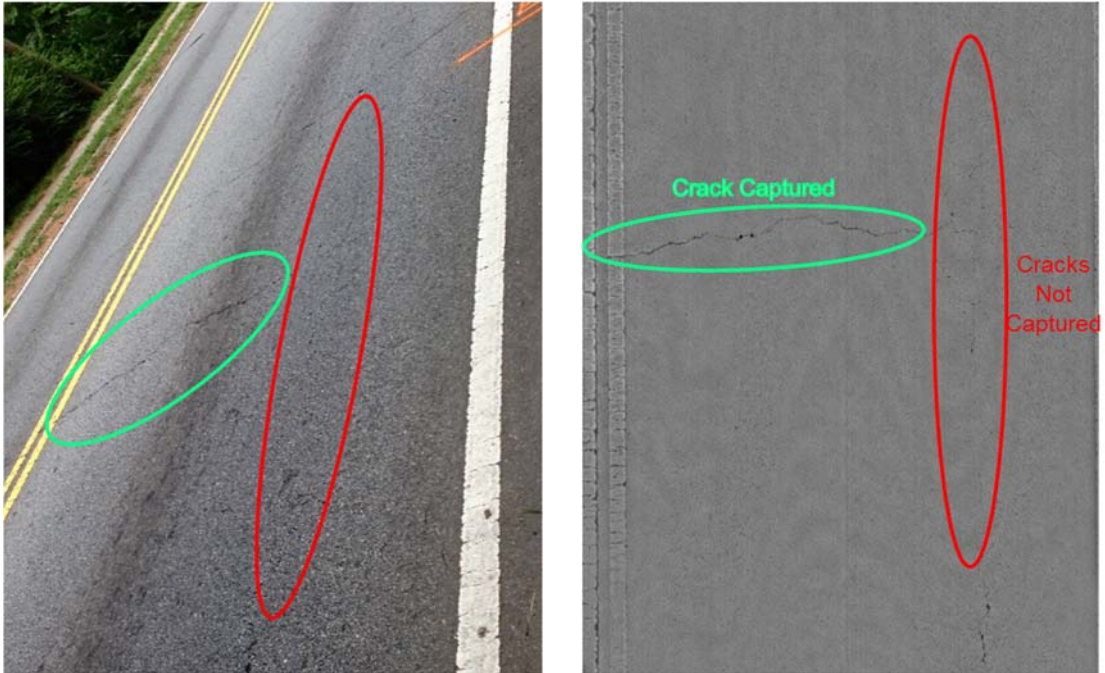
FIGURE 2.5: Limitation of current technology on hairline cracking (images from SR236 Site #3)
