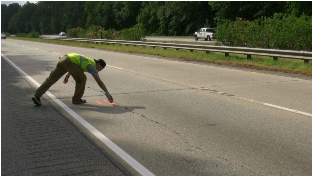
FIGURE 3.2: Manually labeling the selected concrete slab for crack detection validation
