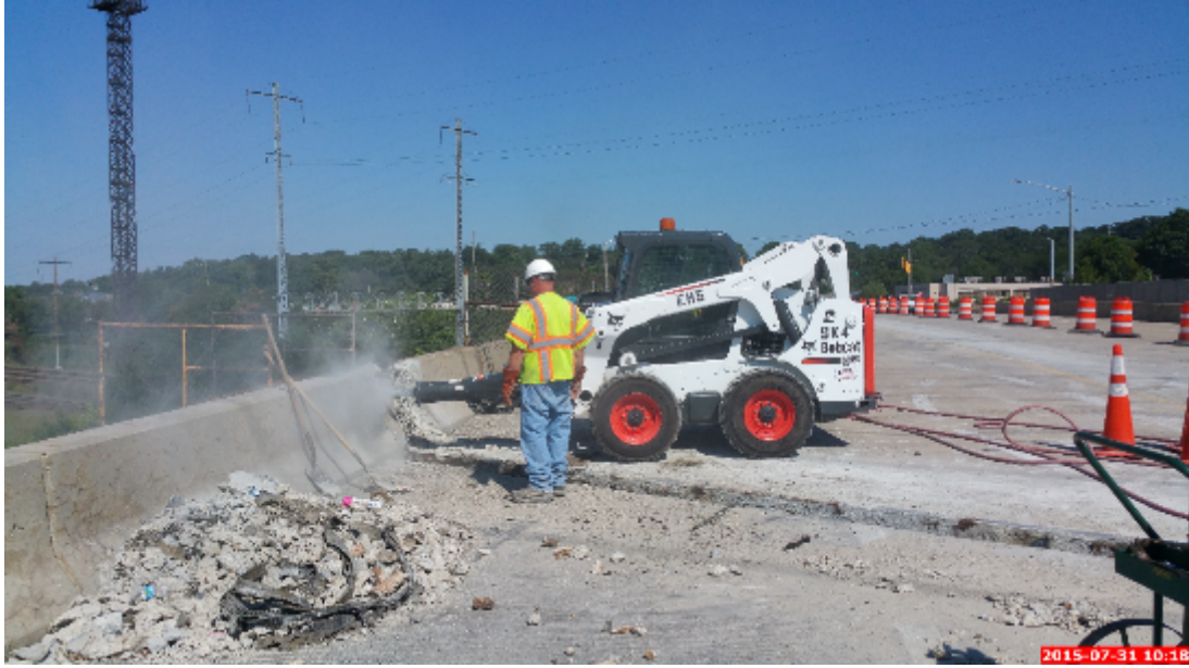
Figure 42: Parapet Body Subjected to Breaking from Skid-Steer-Loader
