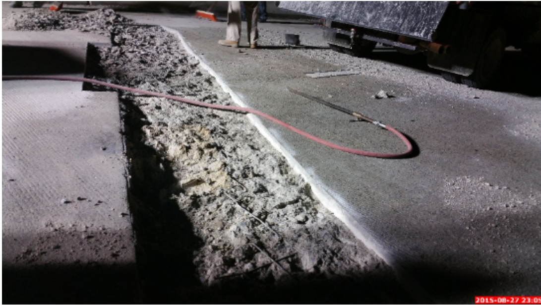
Figure 21: A Deck Patching Operation that Provided a Shallow Depth Concrete Replacement to the Upper Steel Reinforcement Mat
