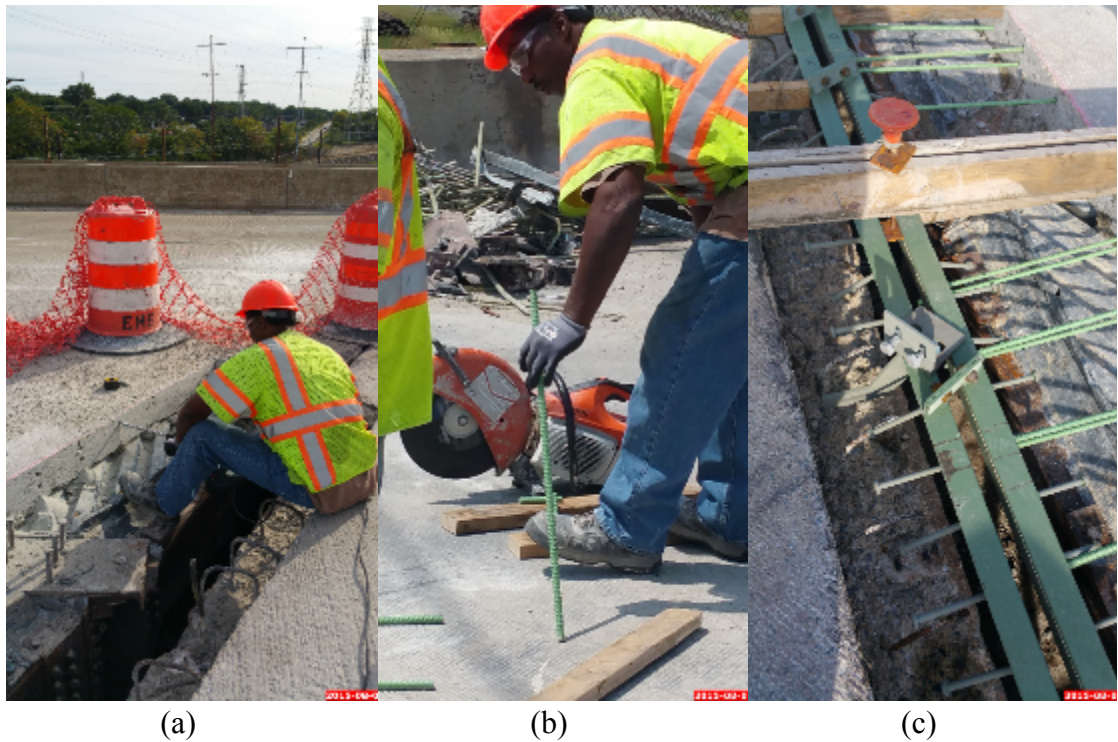
Figure 47: Fitting of the Rebars into the Deck (a) Drilling of the holes for the Dowels, (b) Adjusting the Rebar Length to Fit, and the (c) Placement of the Dowels After the Implementation of the New Armoring System
