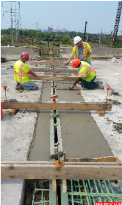
Figure 44: Length Difference Between Pouring and Demolition, the Concrete Held in Place by the “Bulkheads”
