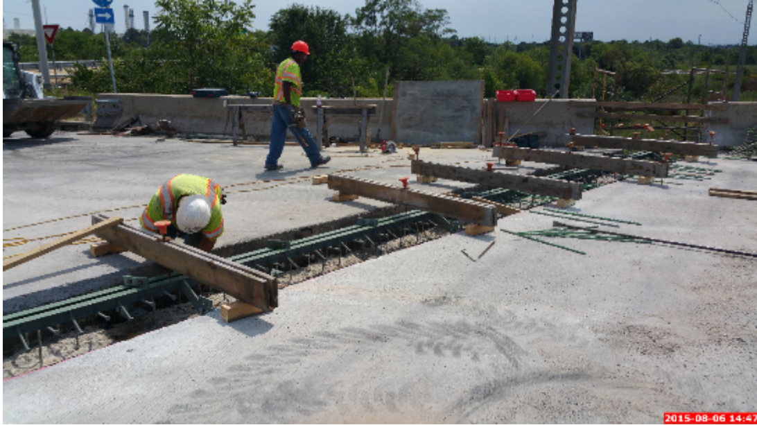
Figure 49: The Temporary Anchorage of the Armoring Systems onto the Deck and Approach Riding Surfaces
