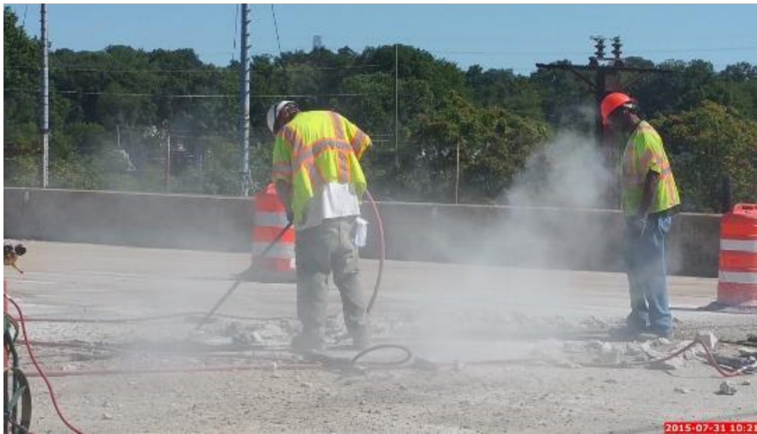
Figure 64: An Example of One of the Many Intermittent Airblasting Session at the End of the First Day of the Demolition Stage
