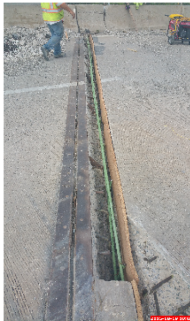
Figure 20: Shallow Depth Removal of North Abutment Backwall Expansion Joint, with Partial Deck Patching in the Surrounding Area
