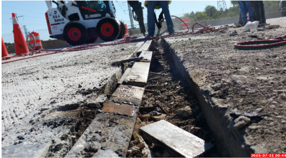
Figure 40: The Skid Steer Loader Breaking on the Deck Header While 30-Pound Breakers Are Utilized on the Backwall
