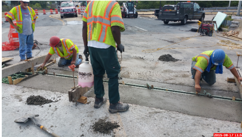
Figure 57: The Smoothing of the Newly Poured Concrete Paired with the Spraying of the Curing Compound
