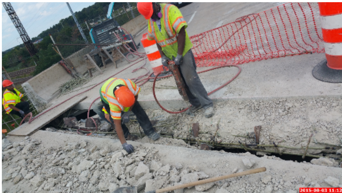
Figure 41: Usage of the 30 Pound Pneumatic Breakers on the Deck Header After Breaking with the Skid Steer Loader Ended
