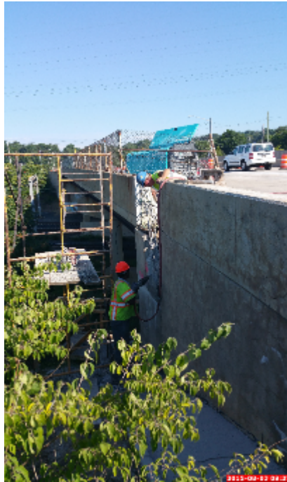
Figure 43: Wing Wall, and the Parapet Base Subjected to Breaking from the Thirty Pound Breaker
