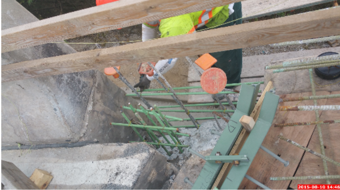
Figure 50: The Intermittent Placement of the Wing Wall/ Backwall Sided Parapet Base Steel Reinforcement
