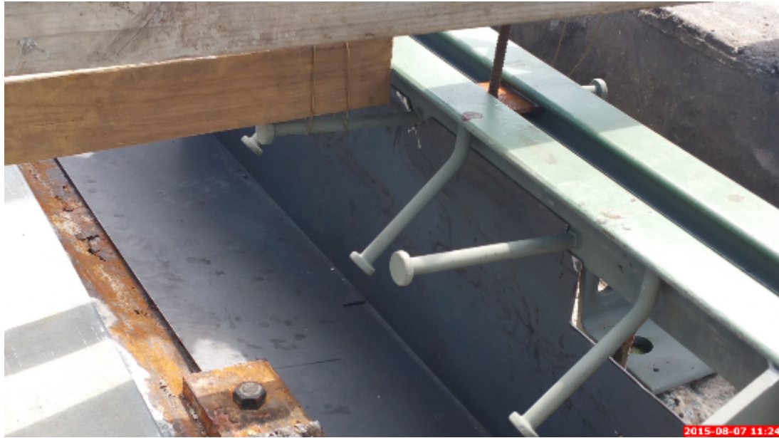
Figure 52: The Metal Formwork Running Along the Pouring Length of the Dam, Connected to the Diaphragm and Bottom Lip of the Armoring
