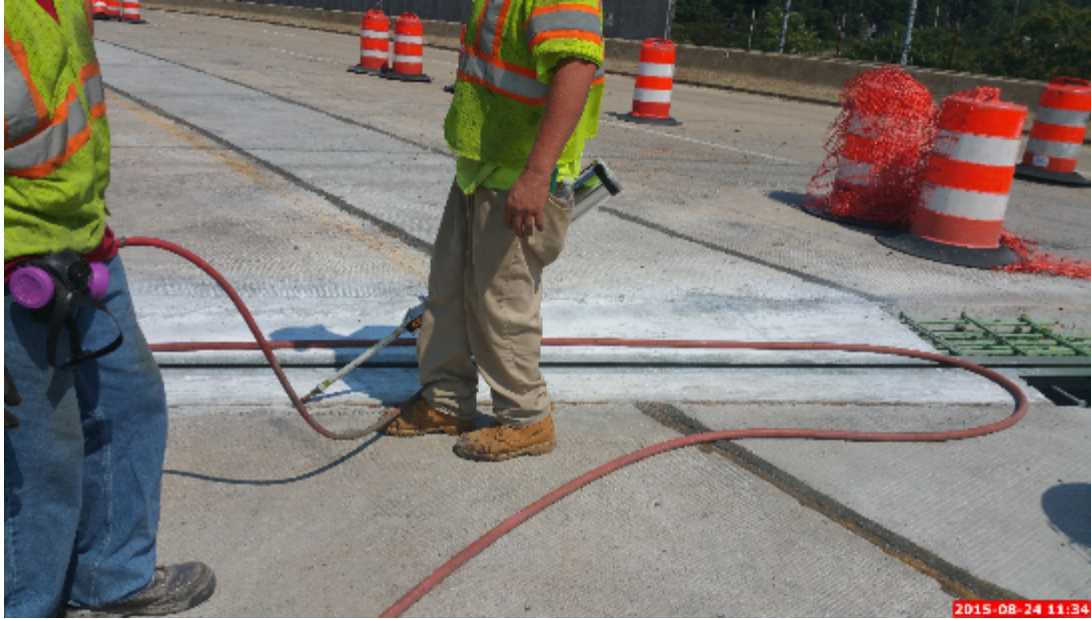
Figure 62: Application of Silicone Within the Backwall and Approach Riding Surface Interface, Above the Cork Formwork
