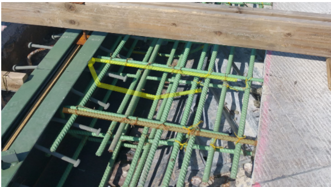
Figure 45: Highlighted in Orange is a Dowel Epoxied into the Deck Wall; Highlighted in Yellow is a Stirrup Tied to its Corresponding Dowel.
