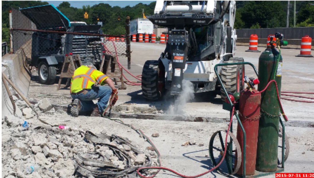
Figure 39: Heat Cutting/Torching Performed Intermittently as Soon as Armoring Elements Made Available to Foreman
