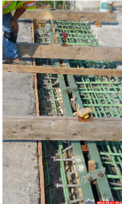
Figure 55: The Cork Formwork Can Be Seen Along the Backwall-Approach Riding Surface Interface, Parallel to the Newly Implemented Rebars
