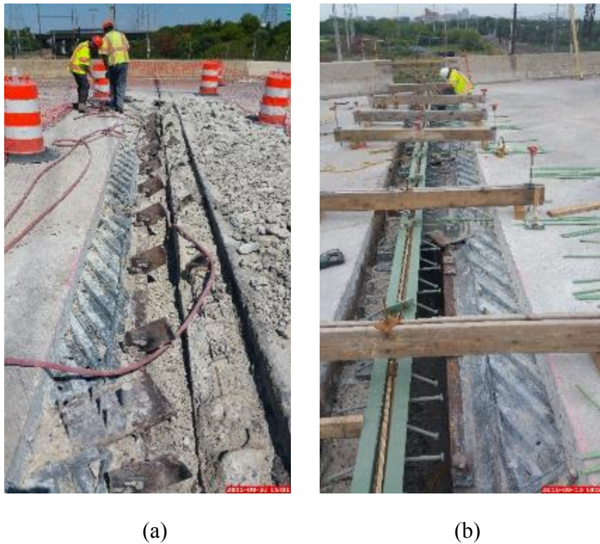
Figure 30: The Reversal of the Anchorage Arrangements from Erection of the Bridge to Reconstruction of the Expansion Joint and Headers -Depiction of Deck Header (10) and Backwall (5) Anchorages Arrangements from (a) Previous Construction and (b) During the Construction Stage
