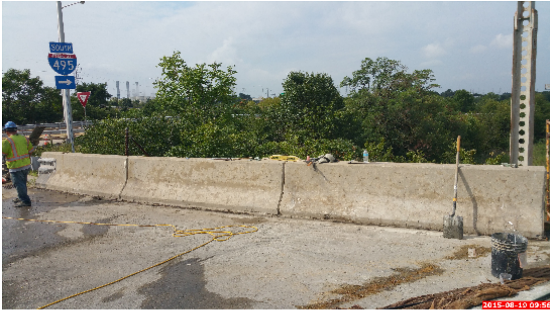
Figure 22: The region of backer rod and silicone between the parapet to approach and backwall header interface to be implemented
