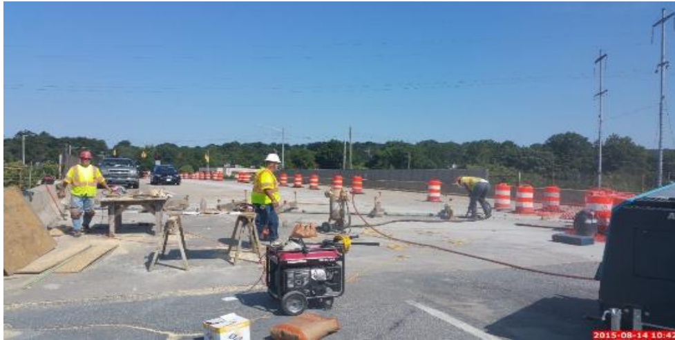
Figure 65: An Example of an Intermittent Sandblasting Session in the Dam In-Between the Placement of the Rebars in the Deck and Backwall Headers
