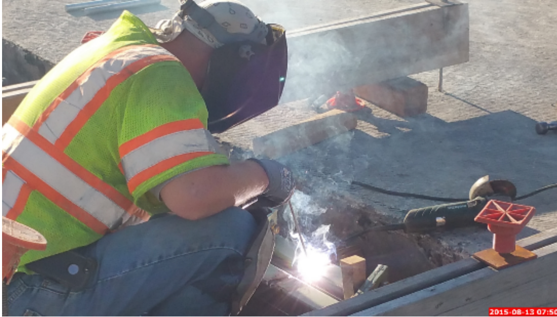
Figure 53: Welding of the Two Separately Delivered and Implemented Armoring Systems to One Another
