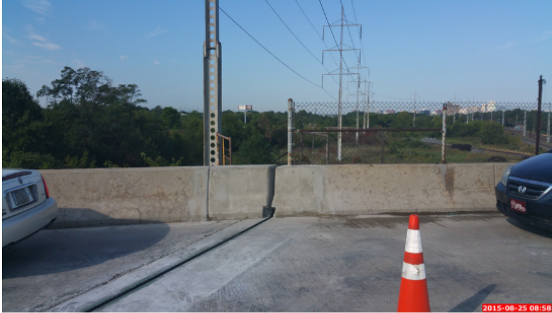
Figure 64: Depiction of Replaced Headers of Lane 1 and the Parapet Resulting from Completion of the Case-Study
