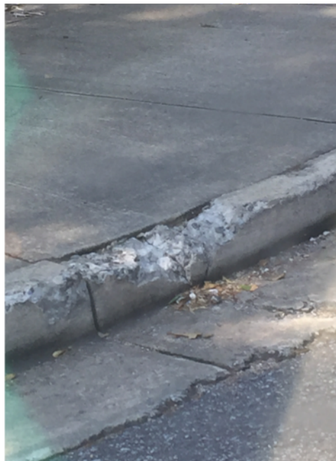
Figure 9-4. Concrete Curb Section Loss
