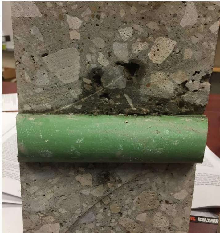
Figure 69 Close-up of tangential core from WAY-30 showing entrapped air voids and moisture penetration above dowel bar.
