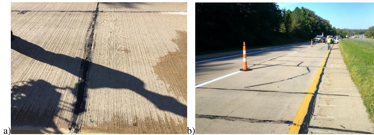
Figure 97 Pavement distress observed on ASD-30, July 8, 2016: a) Joint spalling; b) Longitudinal cracking
