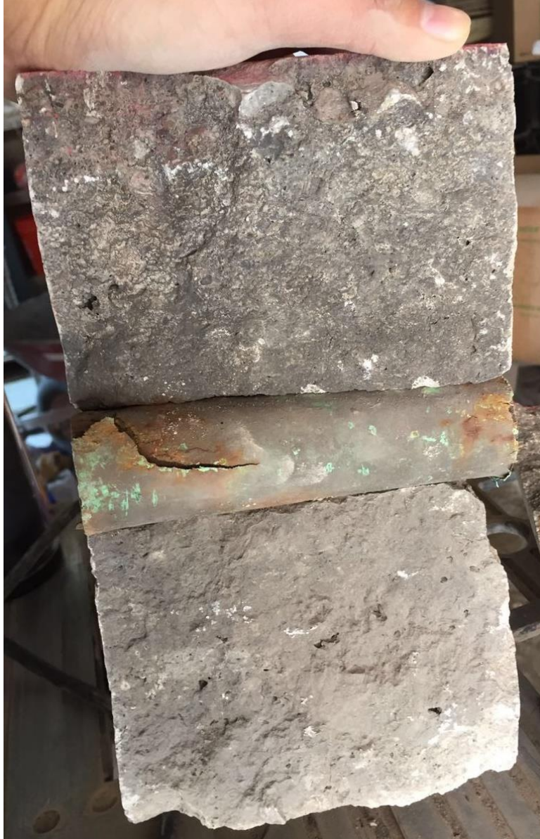
Figure 65 Tangential core with longitudinal crack, opened to show deterioration of concrete, gap above dowel bar, and corrosion of bar.
