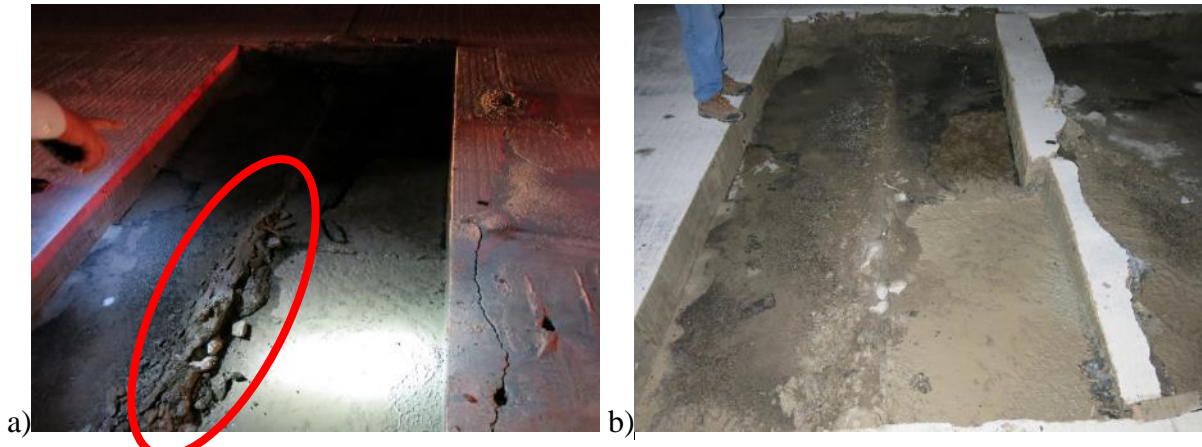
Figure 35 a) Area under segment after removal showing tenting distress (circled); b) Same area under different lighting showing saw slurry from trapped water at lower right.
