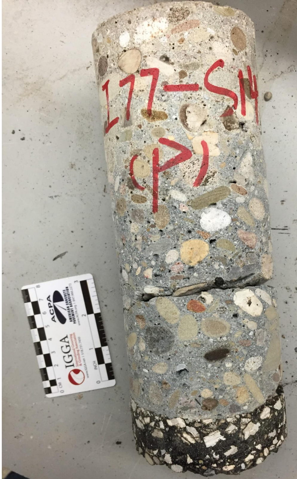
Figure 73 Core with horizontal crack at dowel level from southbound side of WAS/NOB-77.
