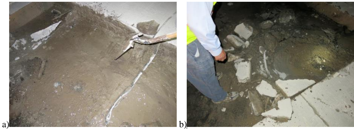
Figure 36 a) Water trapped in the bondbreaker layer; b) Deteriorated bondbreaker
