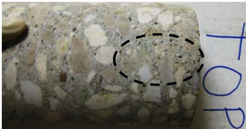
Figure 40 Top-down hairline crack on core W4 from MAD-70 westbound. Photo from report by Dr. Jan Olek of Purdue University.
