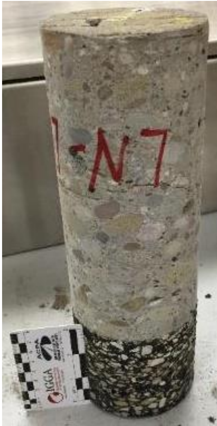
Figure 72 Horizontal crack at dowel level near joint from northbound side of WAS/NOB-77.
