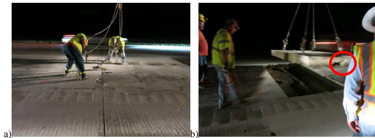
Figure 34 a) Segment being prepared for removal, September 15, 2015; b) Segment being lifted. Circled area shows gap where missing concrete remained in hole.
