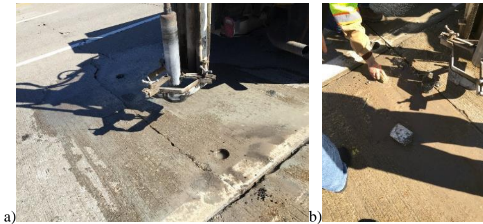
Figure 38 Core holes retaining water.
