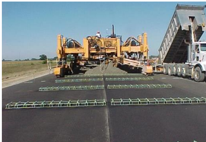
Figure 39 Concrete overlay being placed on a dry bondbreaker surface on MAD-70 in 1999.
