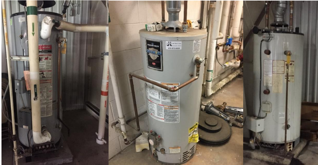
Figure 31 – Existing Standard Efficiency Boilers (Williams, Ottawa, Seneca)
