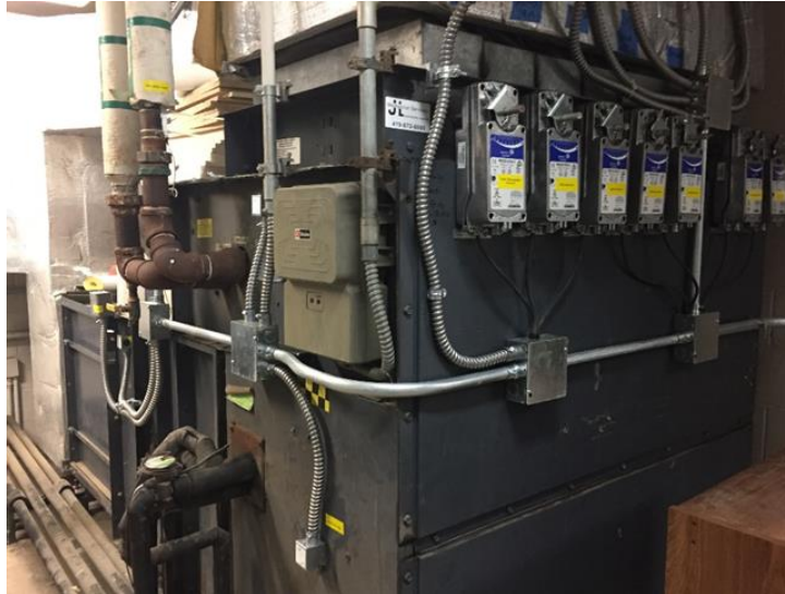
Figure 13 – Ottawa Garage Multi-duct AHU
