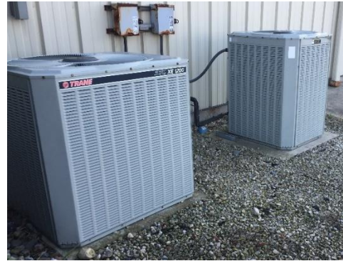
Figure 37 – Seneca Garage Condensing Unit
