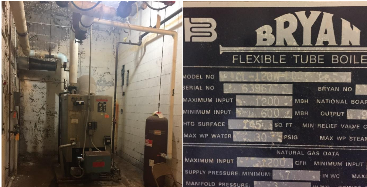
Figure 38 – Headquarters Existing Boiler
