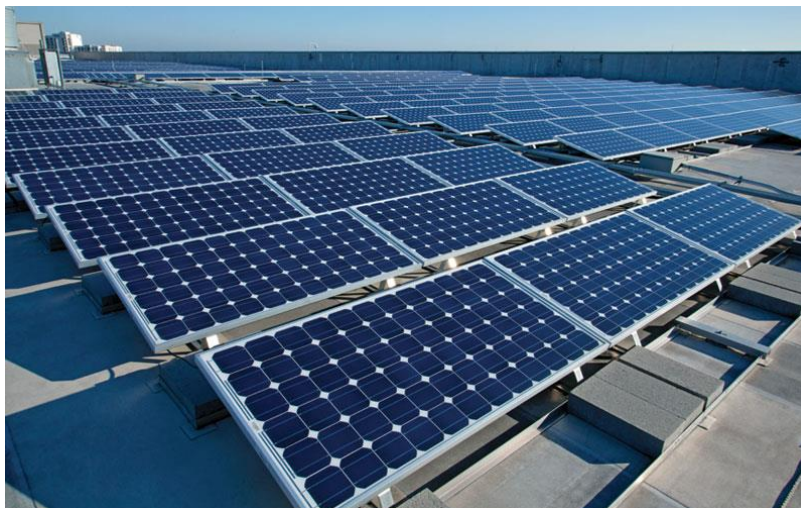
Figure 46 - Roof-Mounted Solar Array
