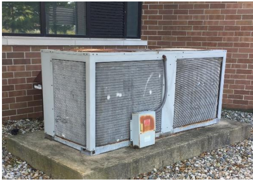
Figure 34 – Ottawa Garage Multi-Duct AHU Condensing Unit
