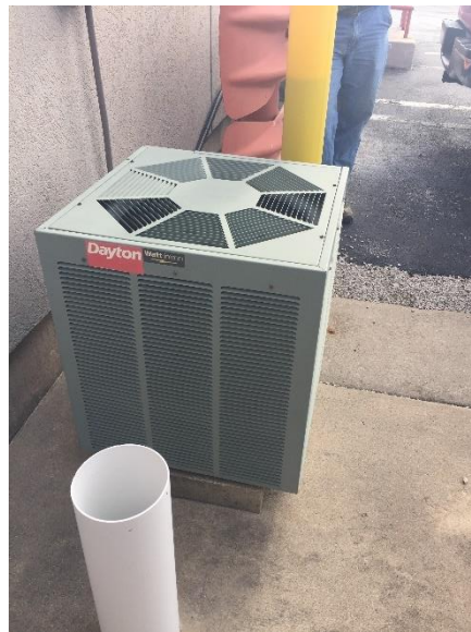
Figure 35 – Headquarters Garage Condensing Unit
