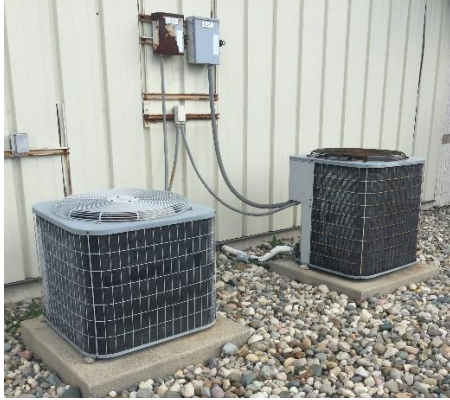
Figure 36 – Williams Garage Condensing Units
