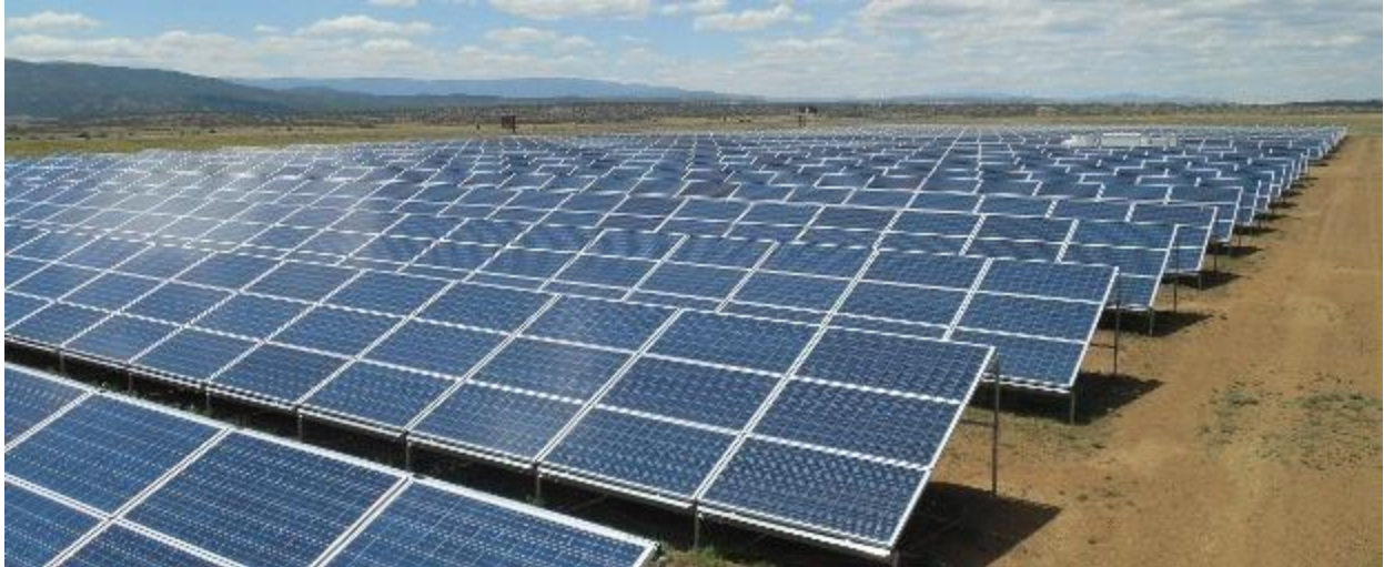
Figure 47 - Ground-Mounted Solar Array
