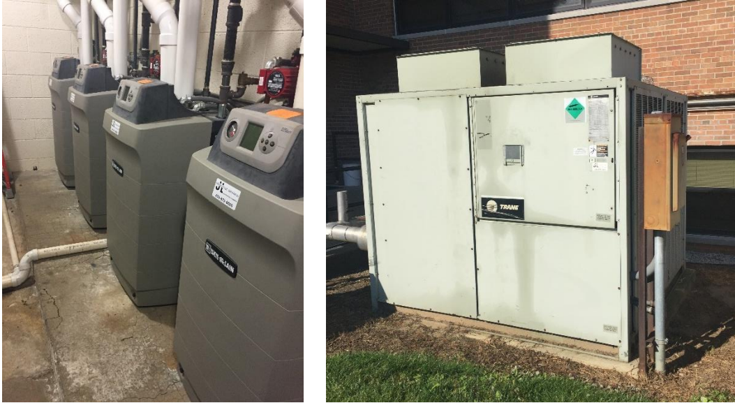
Figure 5 – HQ Office Building Boilers and Condensing Unit
