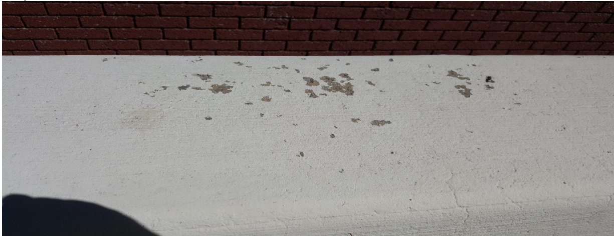
PolyCarb 58.6 – (B), (LM) Delamination on horizontal. Vertical intact.
