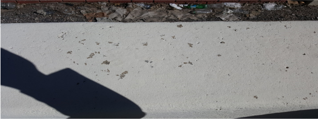
PolyCarb 58.6 – (UB), (LM) Delamination on horizontal
