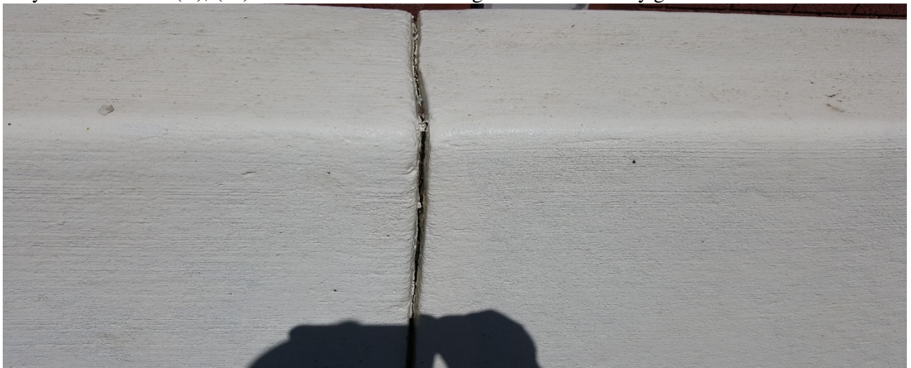
PolyCarb 124/73 – (B), (W) No delamination. Coating intact. Looks very good.
