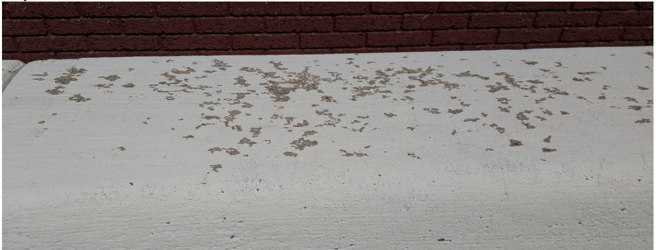
PolyCarb 58.6 - (B), (W) Delamination on horizontal.
