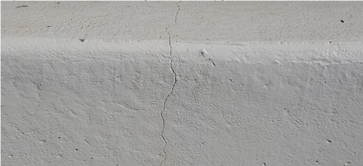
PolyCarb 124/73 – (UB), (LM) Coating intact. Looks very good.
