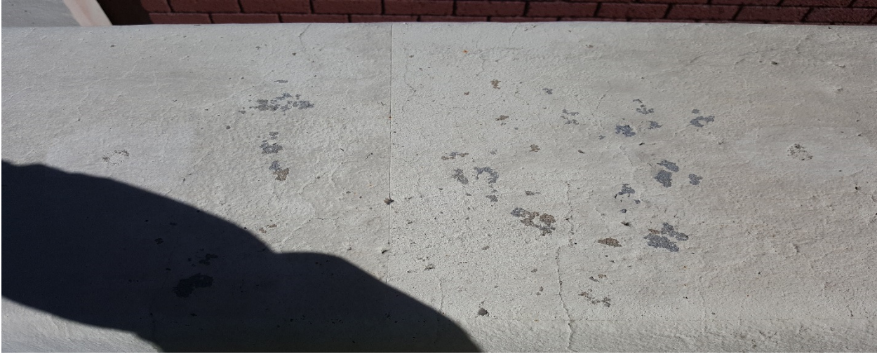
Klaas Coatings – (UB), (LM) Delamination on the horizontal. Vertical intact.
