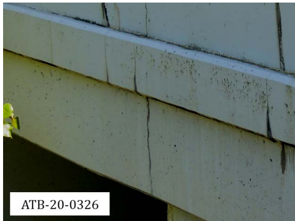
Fig. 3 Nearly Full-Depth Flexural Cracks
