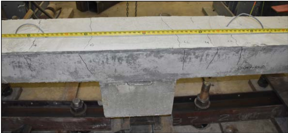
Figure G.20 Cracks in Specimen with a Rigid Connection
