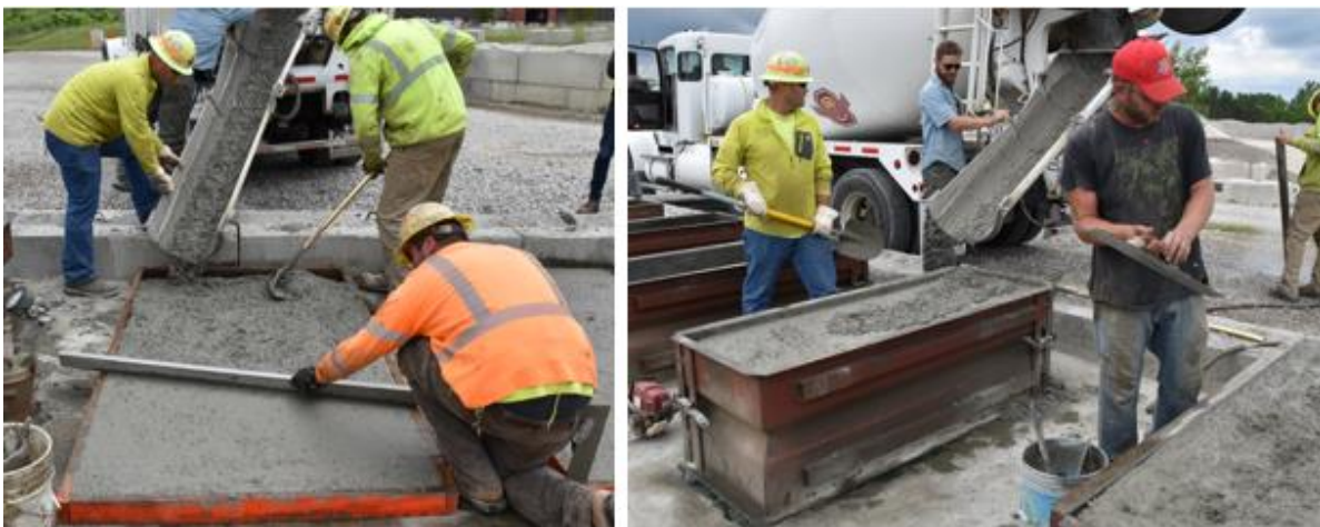
Figure H.7 Placement of Concrete into the Formwork for Slab 2 and Deep Shoulder Benches
