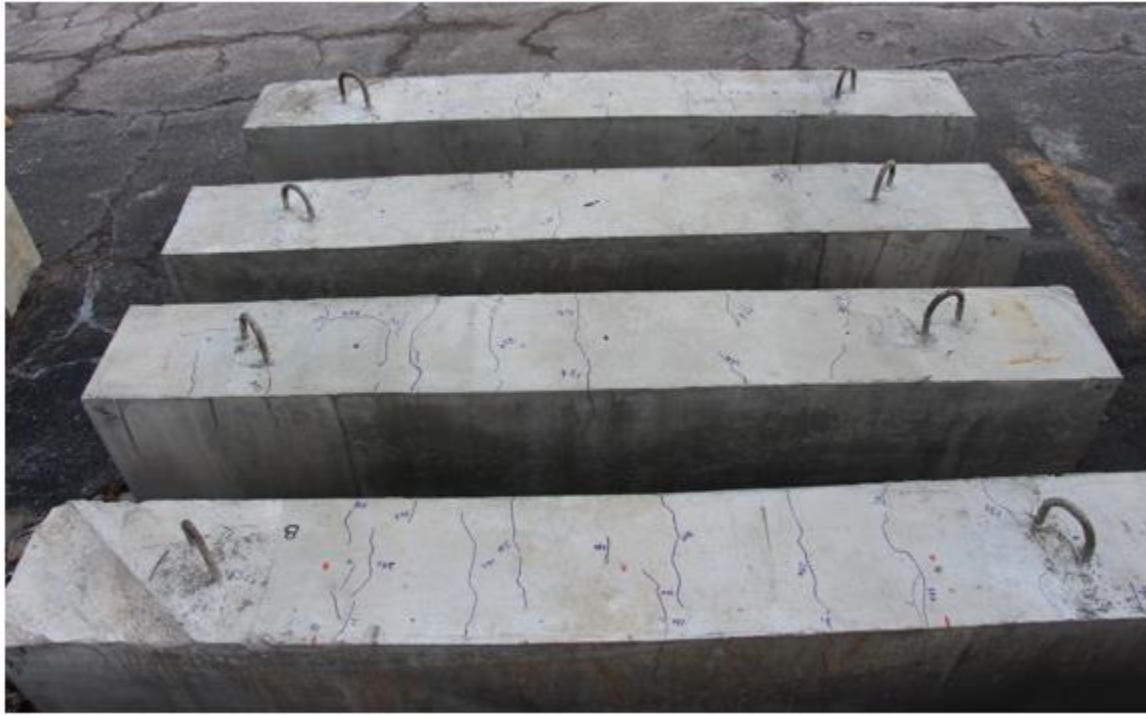
Figure F.43 Crack Patterns on Slabs with Black Bars and Epoxy-Coated Bars ( Black Bars in Foreground and Epoxy-Coated Bars in the Back )
