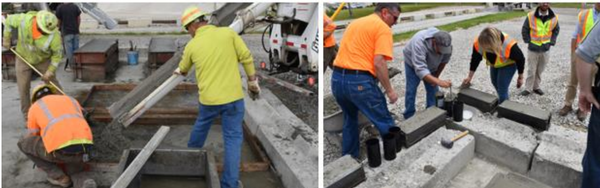
Figure H.6 Placement of Concrete into the Formwork for Slab 1 and Beams
