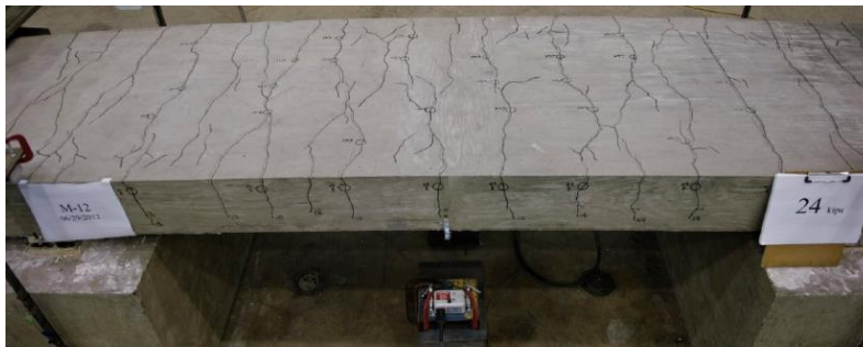
Figure A.29 Cracks Developed in the Constant Moment Region of the Slab
