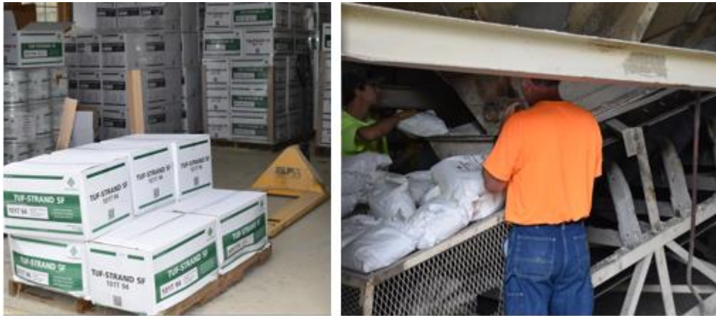
Figure H.2 Euclid TUF-Strand SF 101T94 (left) and Placement of Fibers on Conveyor at the Batching Plant (right)
