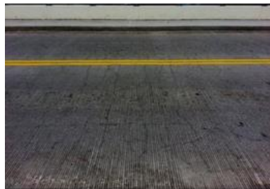
Figure F.32 Bridge POR-88-1250: Transverse Sectional Details (Top), Observed Cracks (Bottom)
