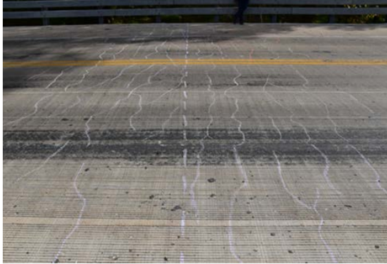
Fig. 6 Severely Cracked Bridge Deck
