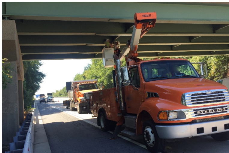
Figure D-6: Hands-on inspection of steel girders and bracings of the bridge
